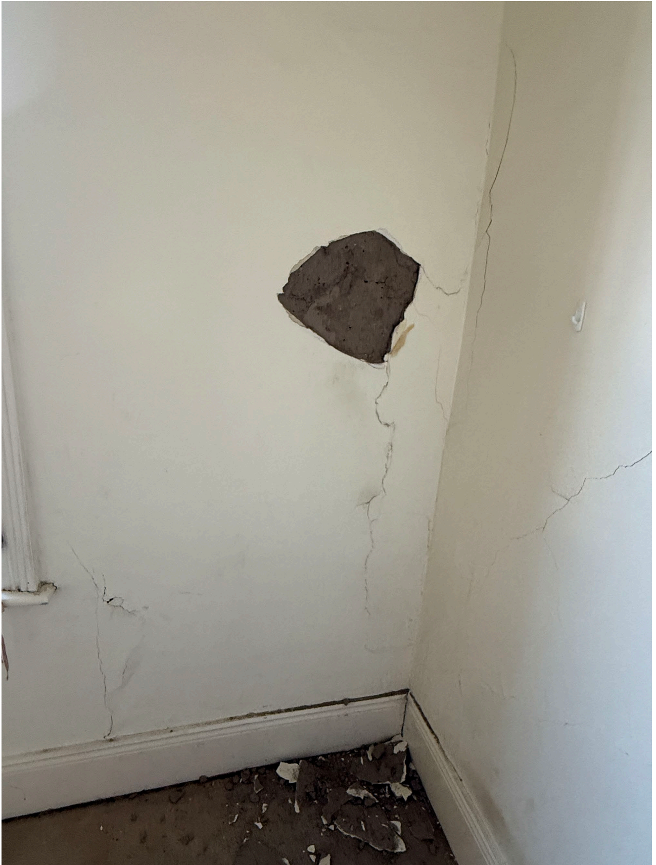
Internal 15 (Damage category 3)
