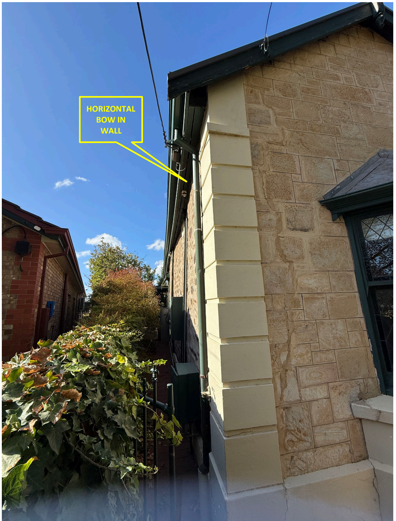
North western wall 08 (Damage category 4)
