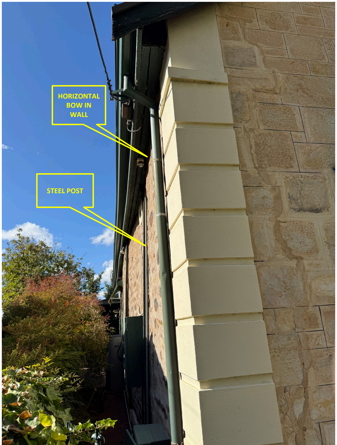
North western wall 09 (Damage category 4)
