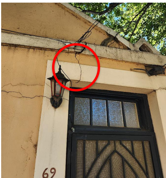
Vertical cracking above entry door.
