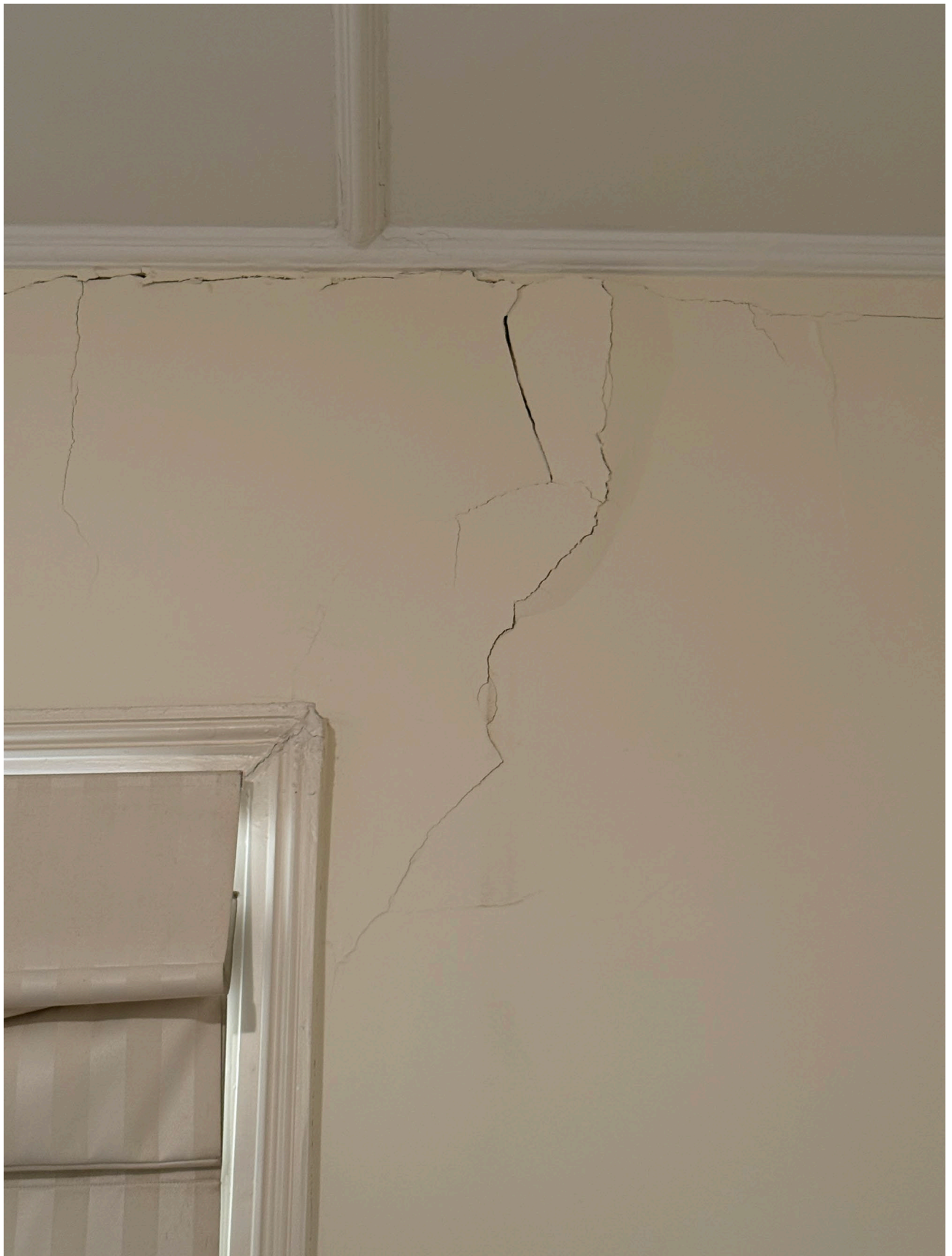
Internal 08 (Damage category 3)
