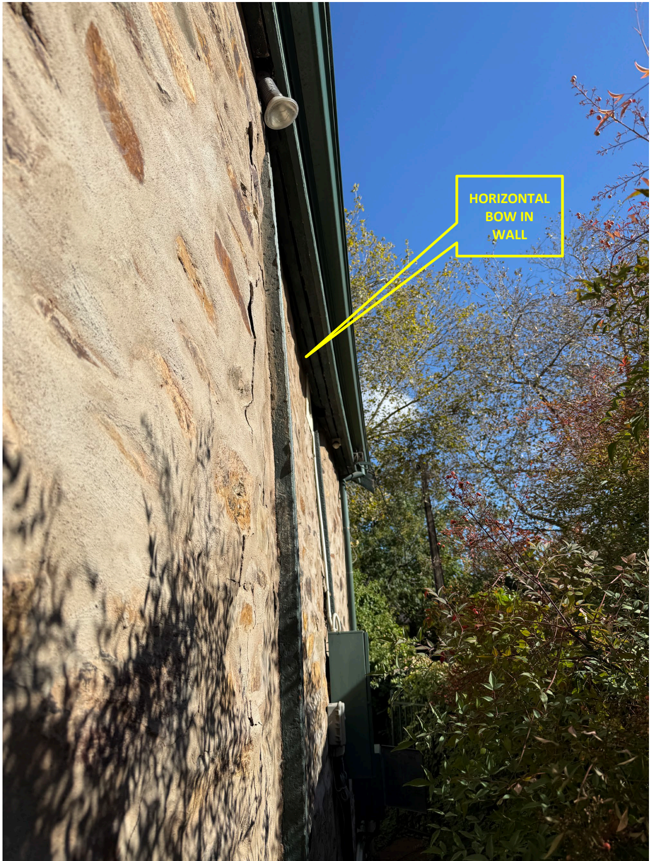
North western wall 02 (Damage category 4)
