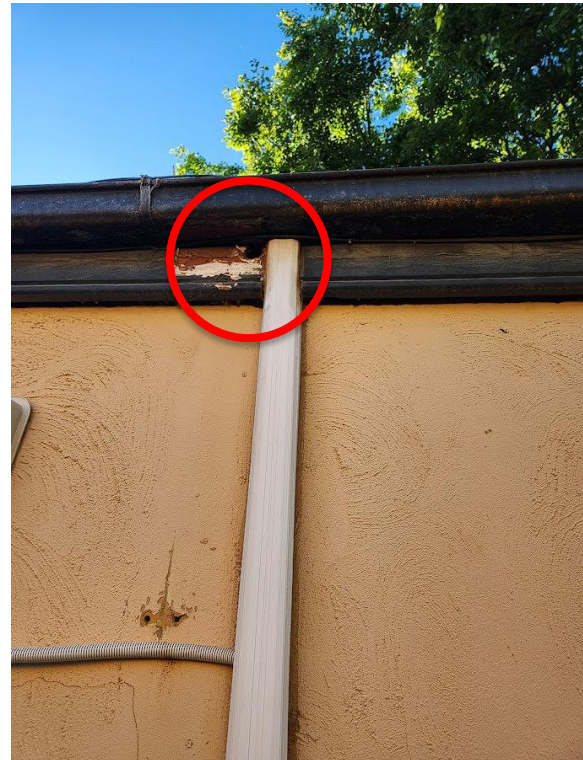
Holes in fascia board.
