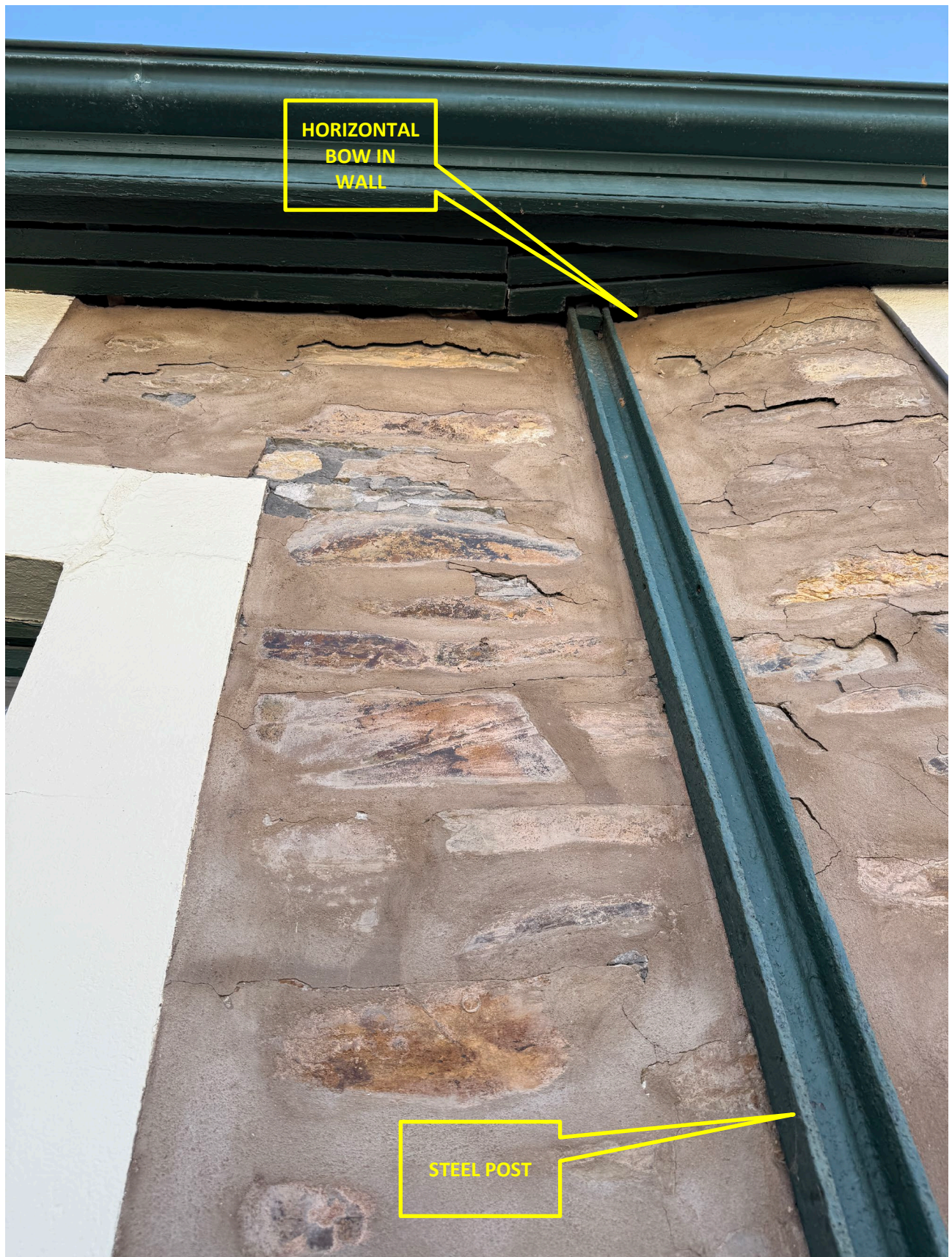
South eastern wall 01 (Damage category 4)
