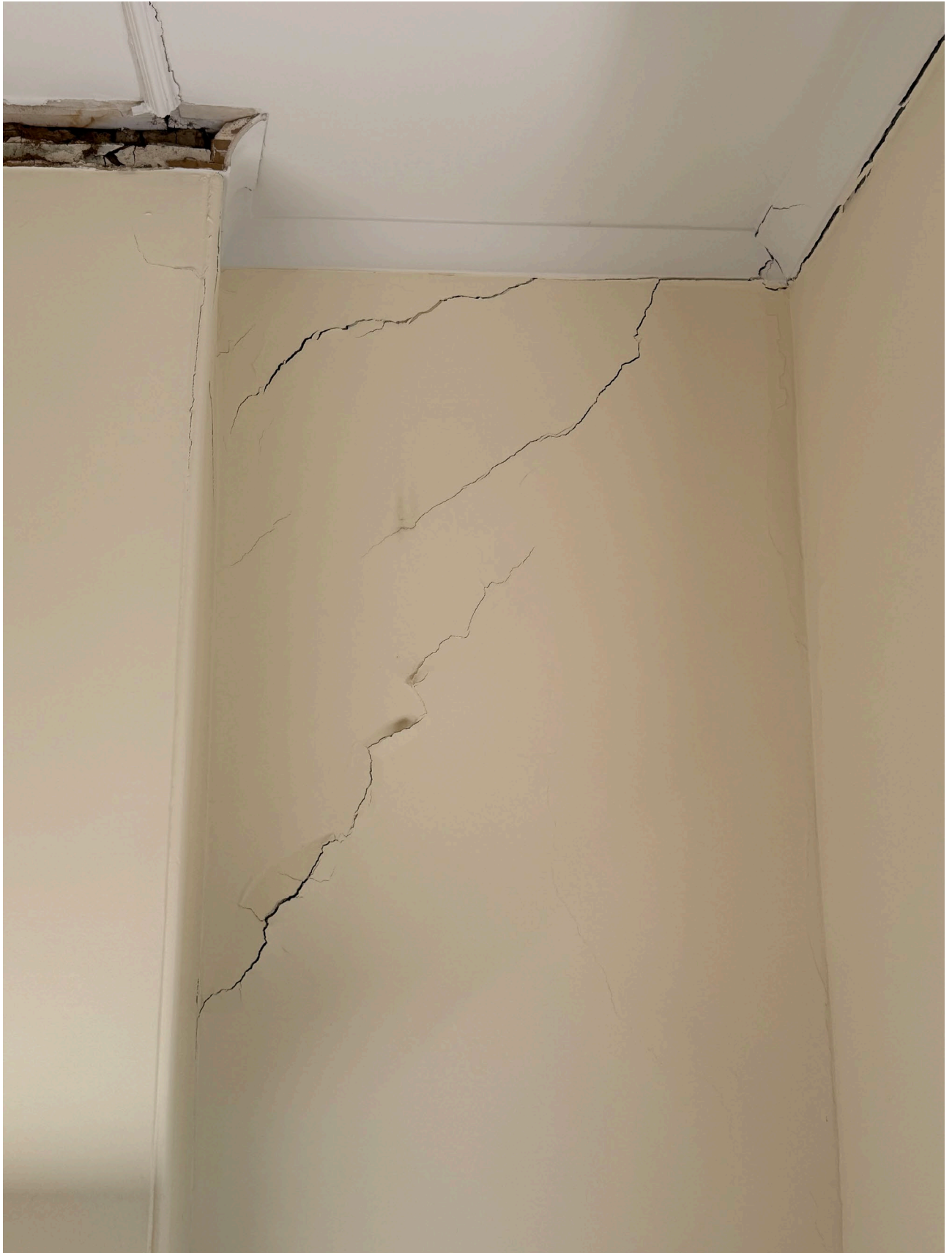
Internal 12 (Damage category 4)
