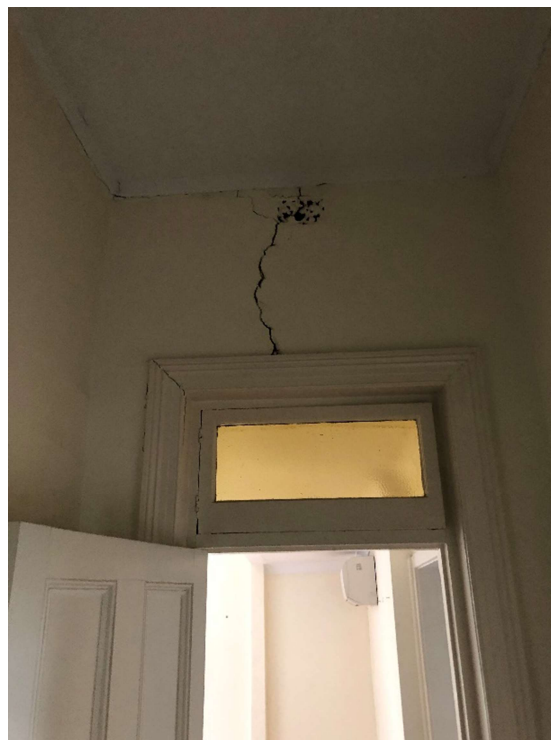
12. Internal view Major cracking and deformation
