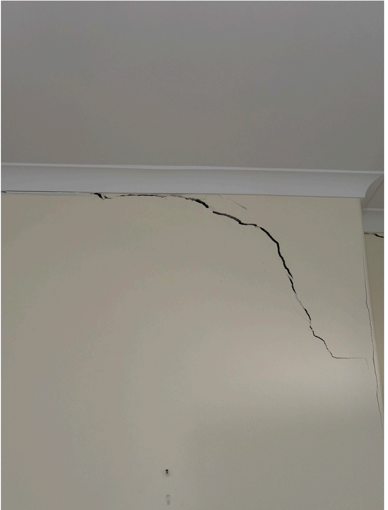
Internal 05 (Damage category 3)
