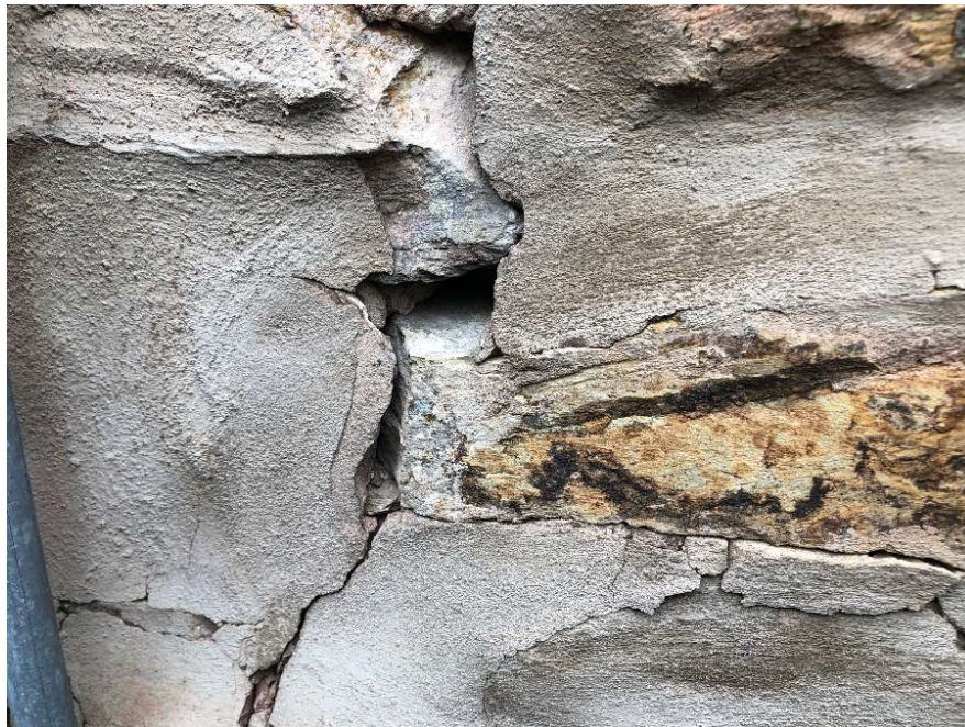
6. North west wall. Severe cracking in masonry wall
