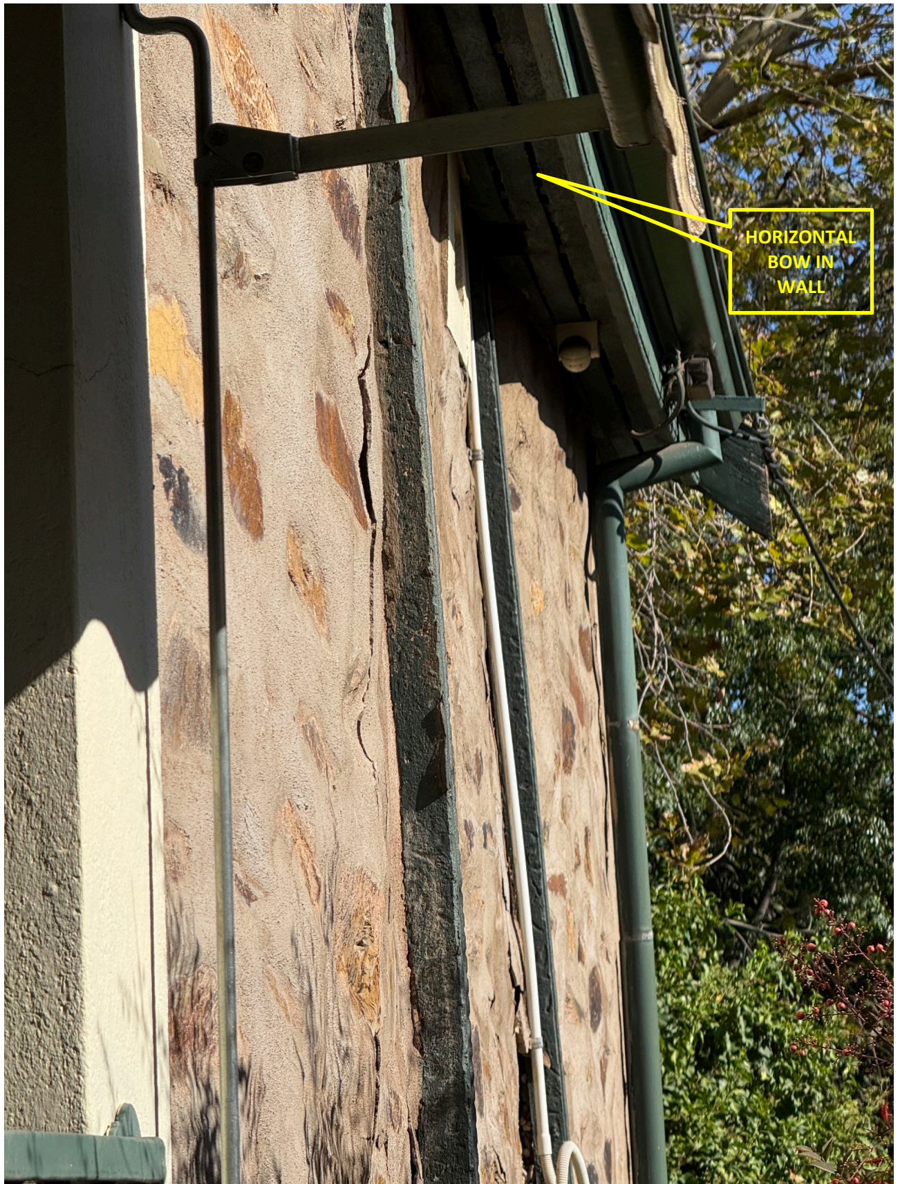
North western wall 03 (Damage category 4)
