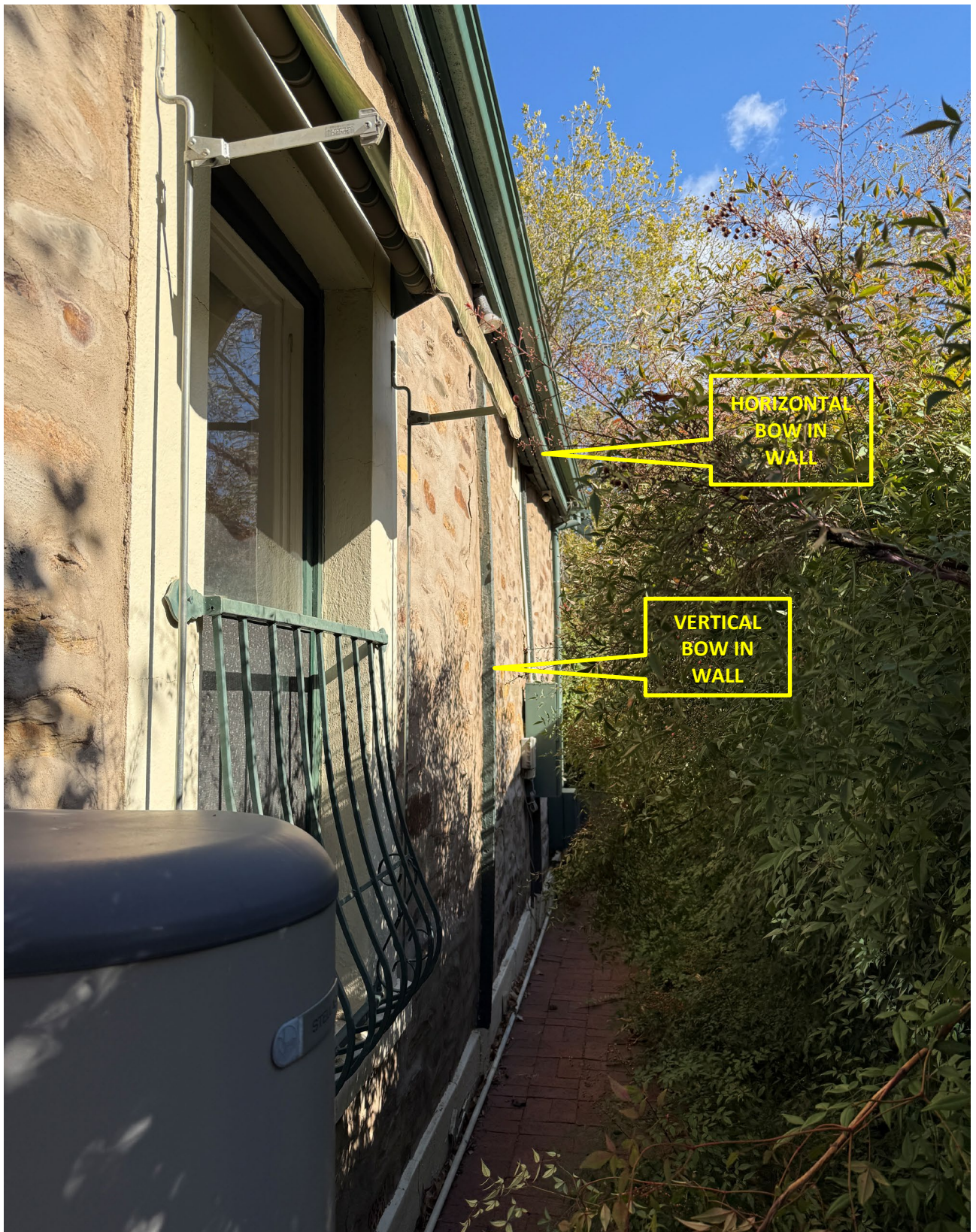
North western wall 01 (Damage category 4)
