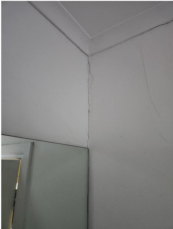
Vertical cracking in northeastern corner of room.
