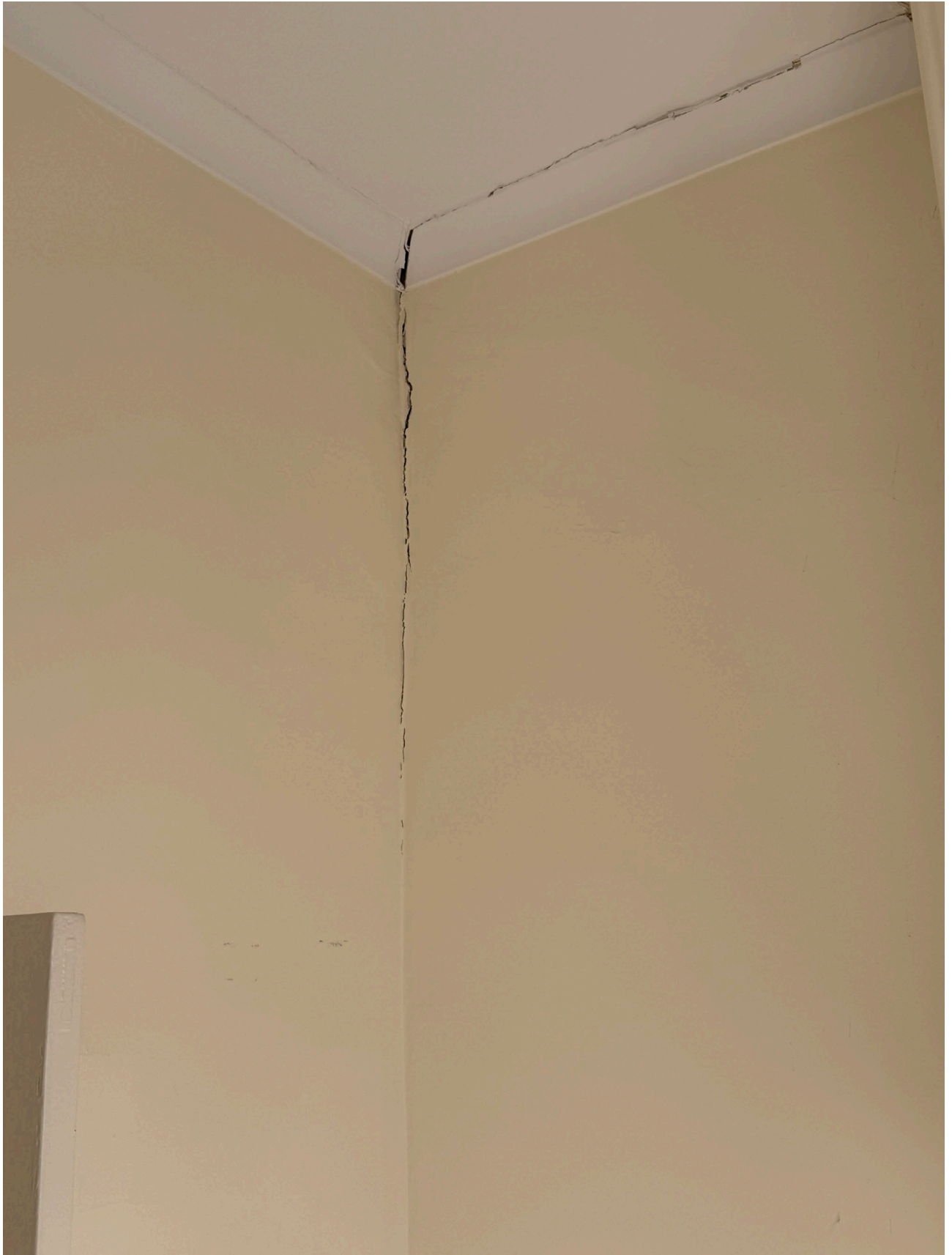
Internal 13 (Damage category 2)
