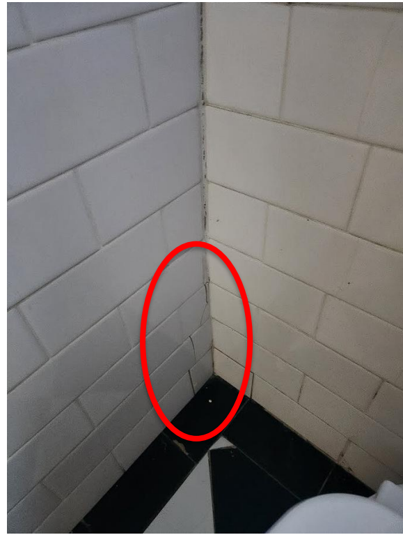
Broken tiles in southwestern corner of room.
