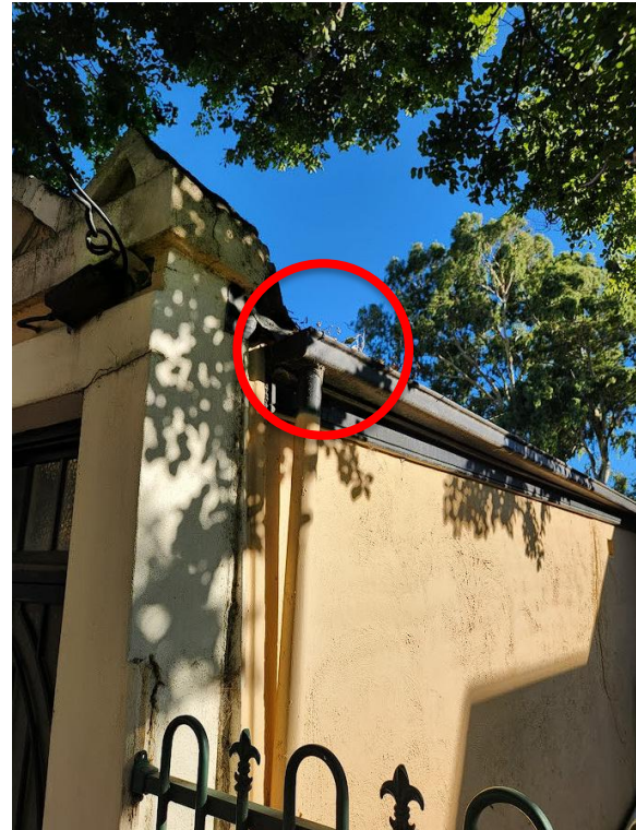
Debris in gutter.
