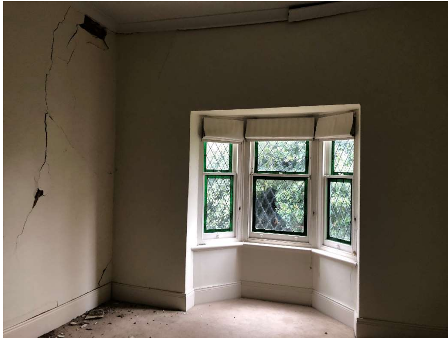
7. Internal view, front room. Cracking in internal wall and cornice.
