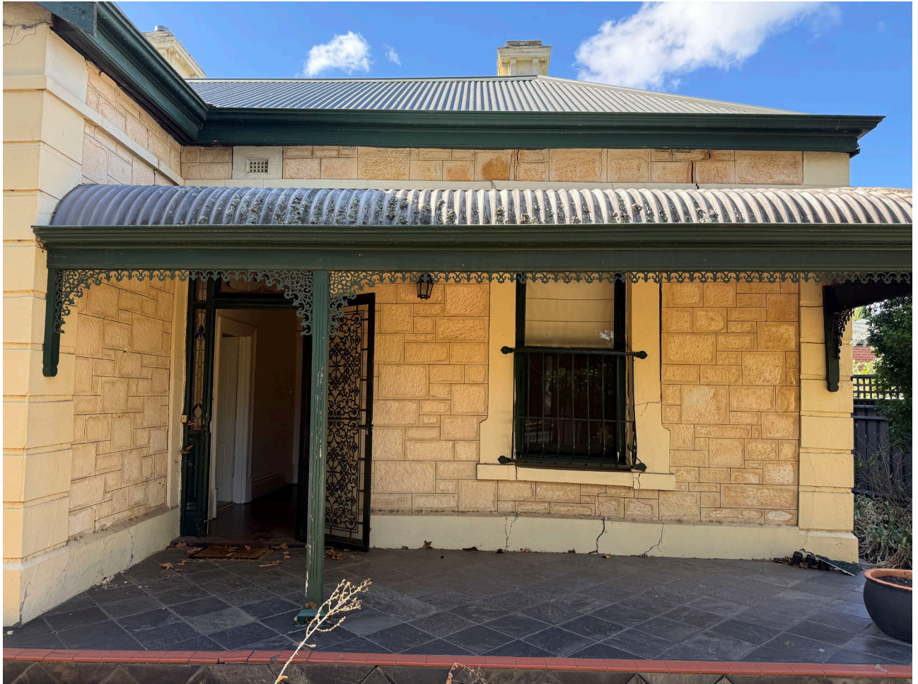
Front wall 01 (Damage category 3)
