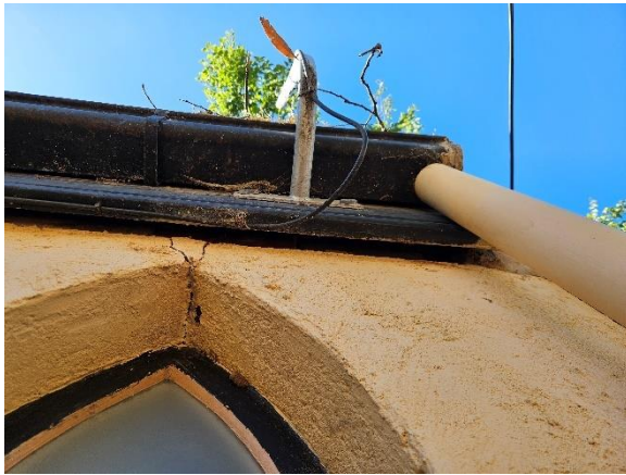
Photo 11 – Separation between western elevation and fascia
