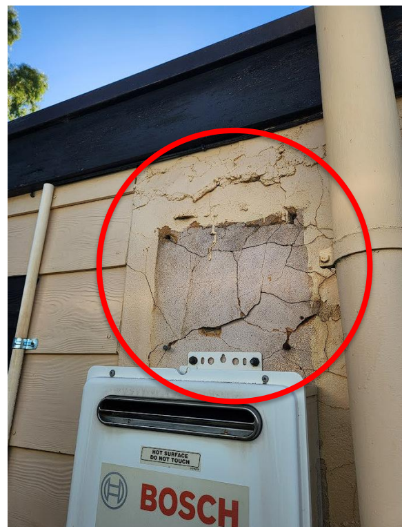
Cracking to render above water heater.
