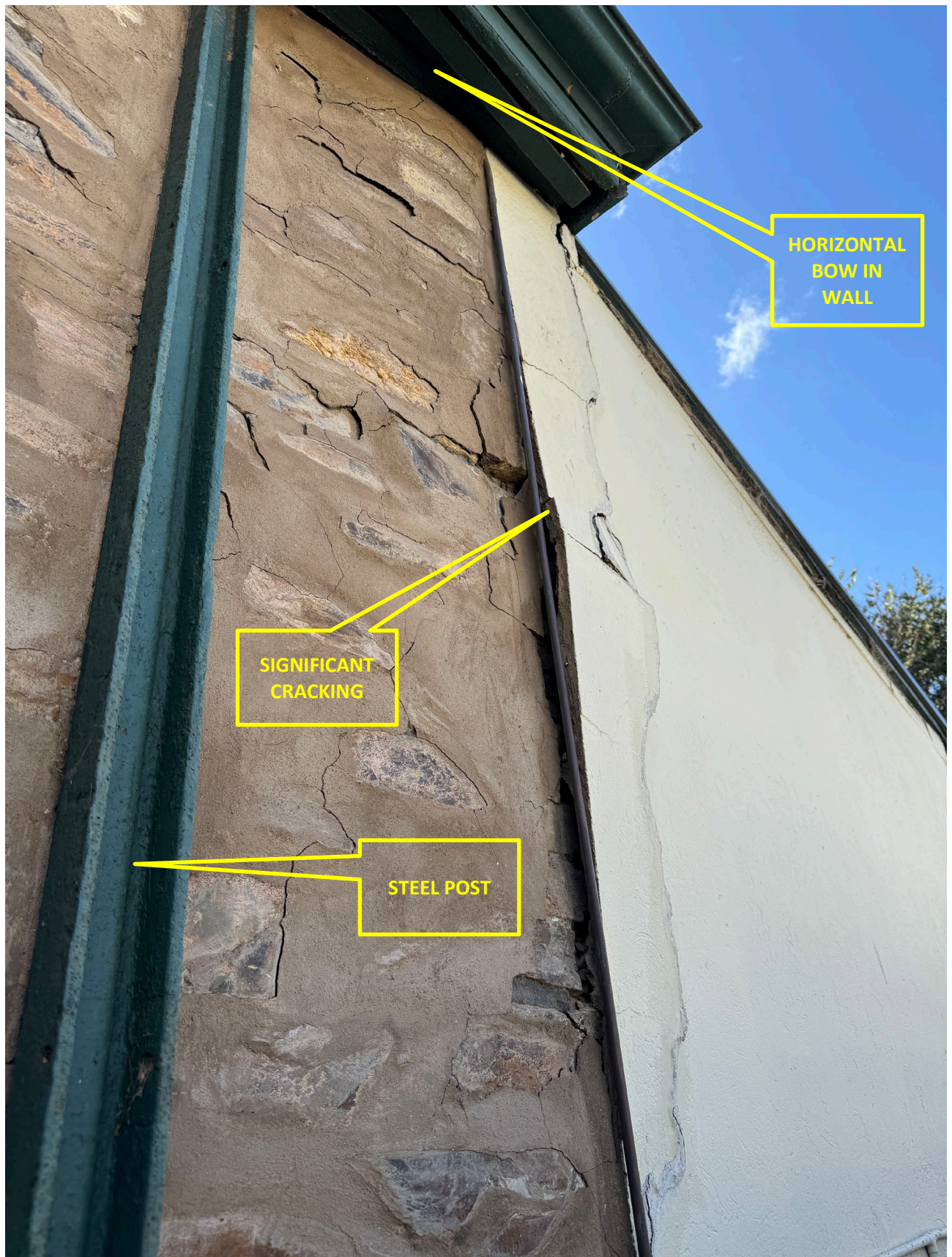
South eastern wall 01 (Damage category 4)
