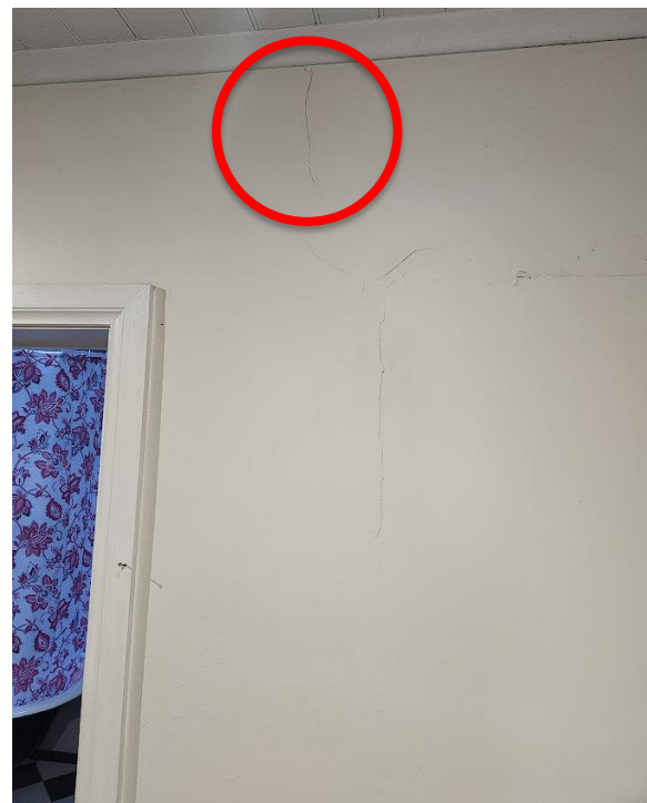
Vertical cracking to northern wall of room.
