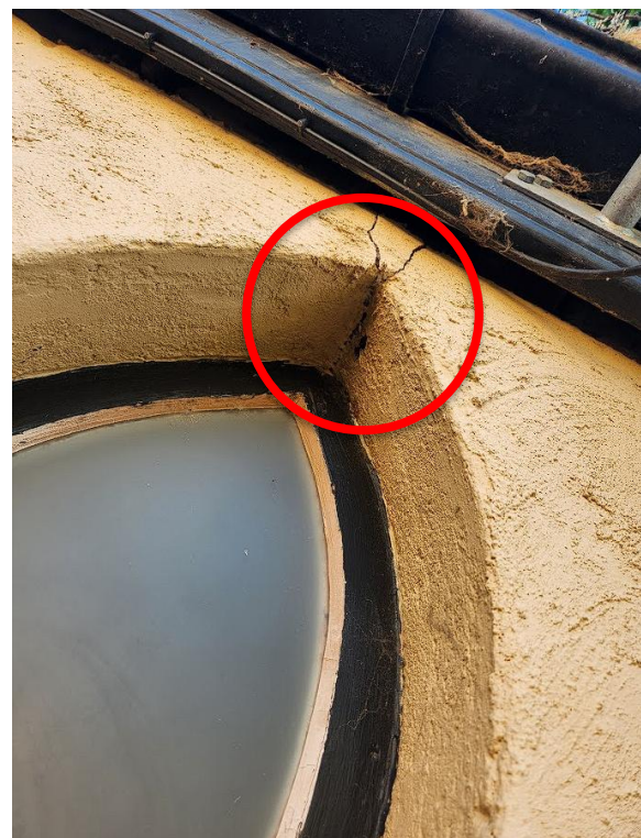
Cracking above western lounge room window.
