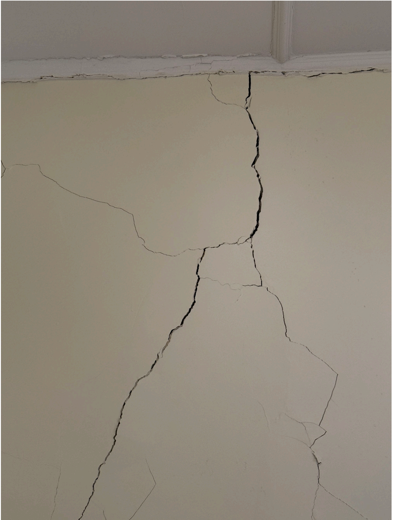
Internal 11 (Damage category 4)
