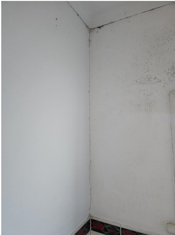
Vertical cracking in southwestern corner of room.
