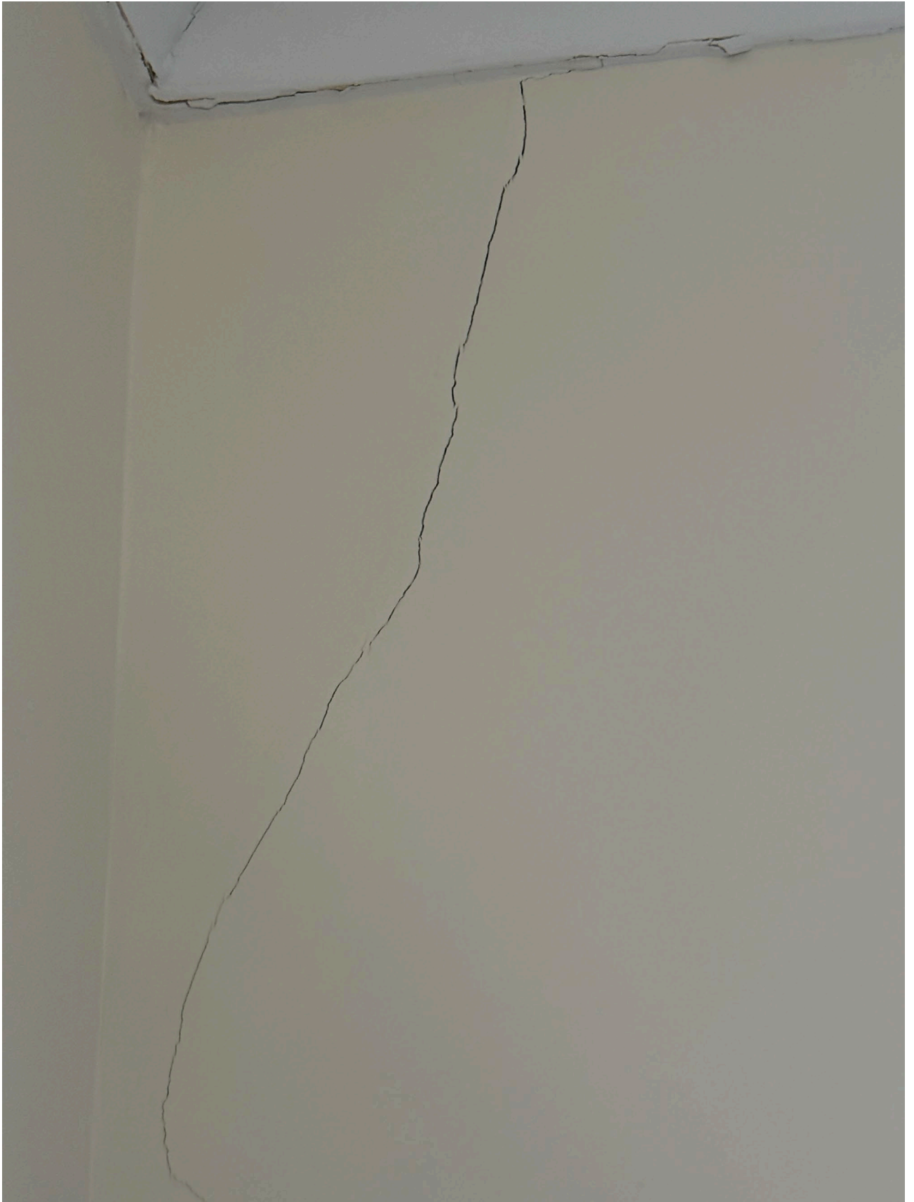
Internal 16 (Damage category 3)
