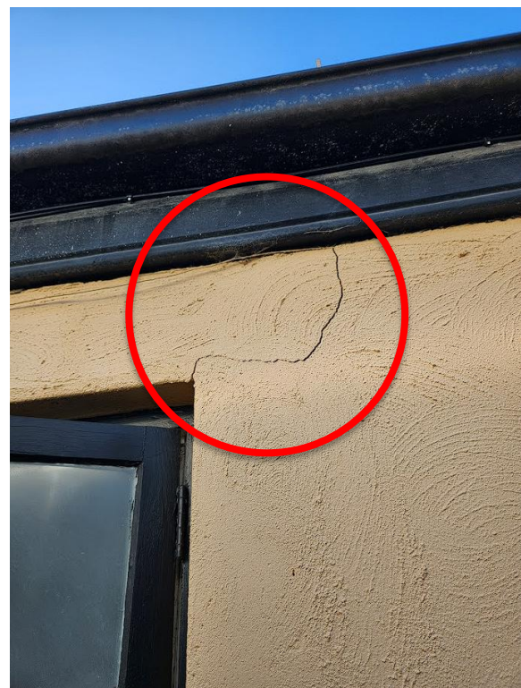
Diagonal cracking above kitchen window.
