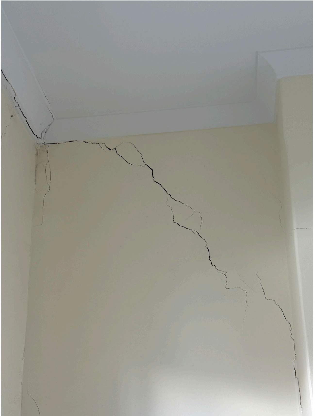
Internal 14 (Damage category 4)
