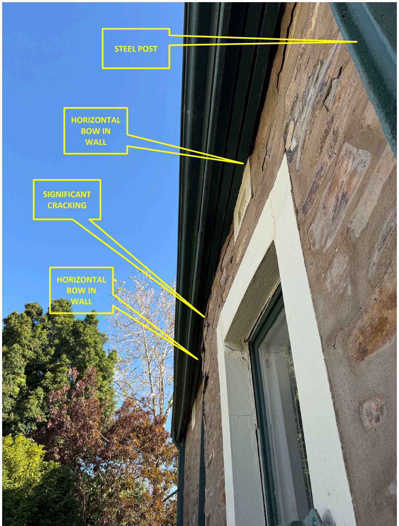
South eastern wall 01 (Damage category 4)
