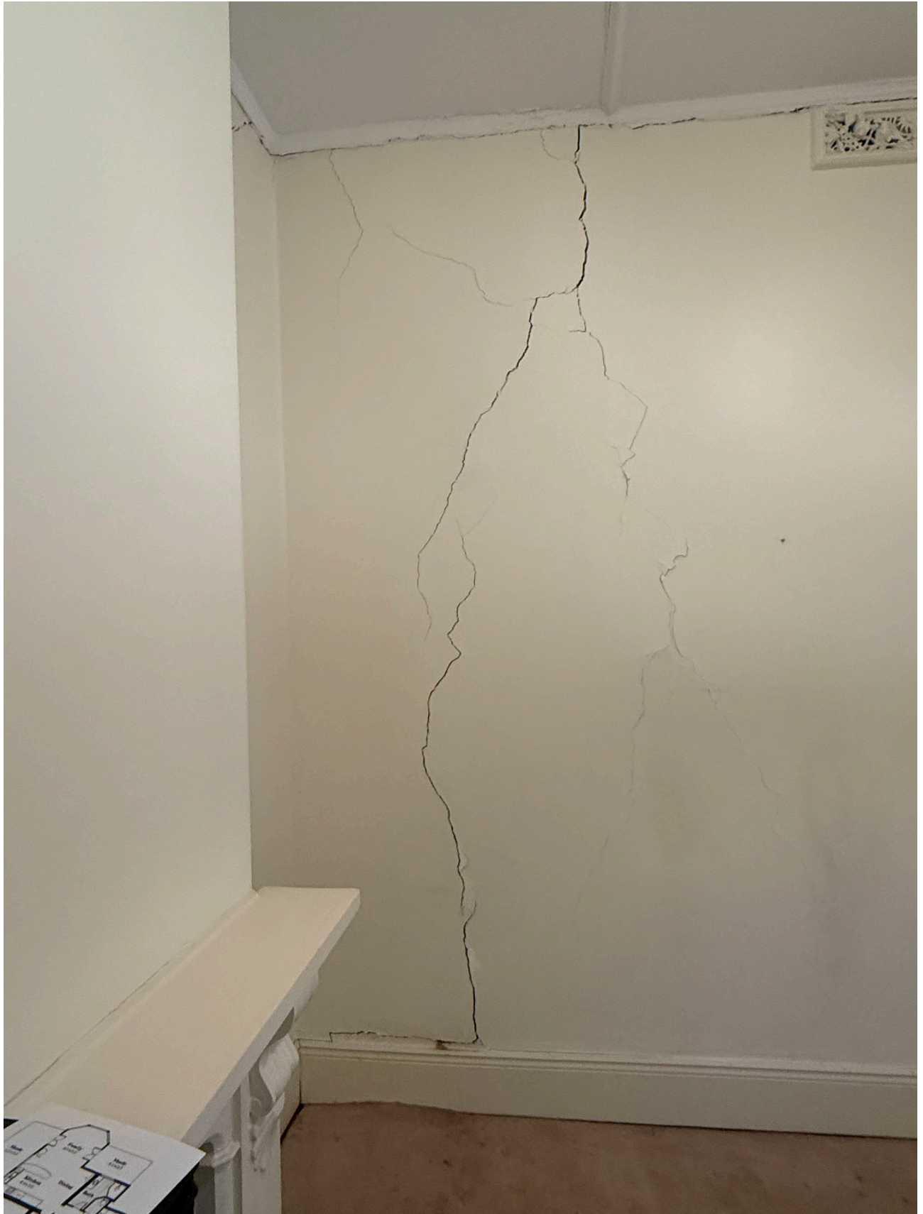
Internal 10 (Damage category 4)
