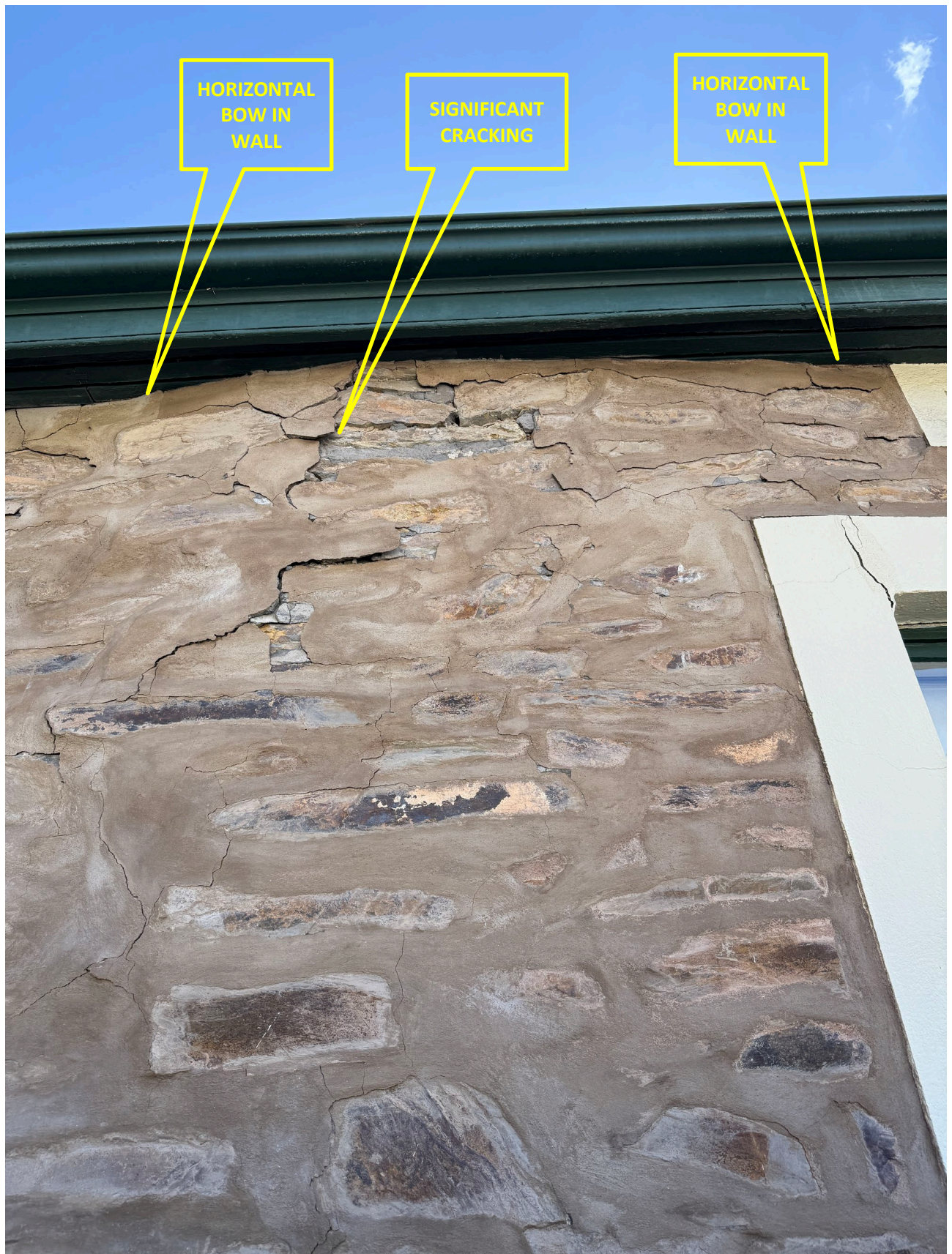
South eastern wall 01 (Damage category 4)
