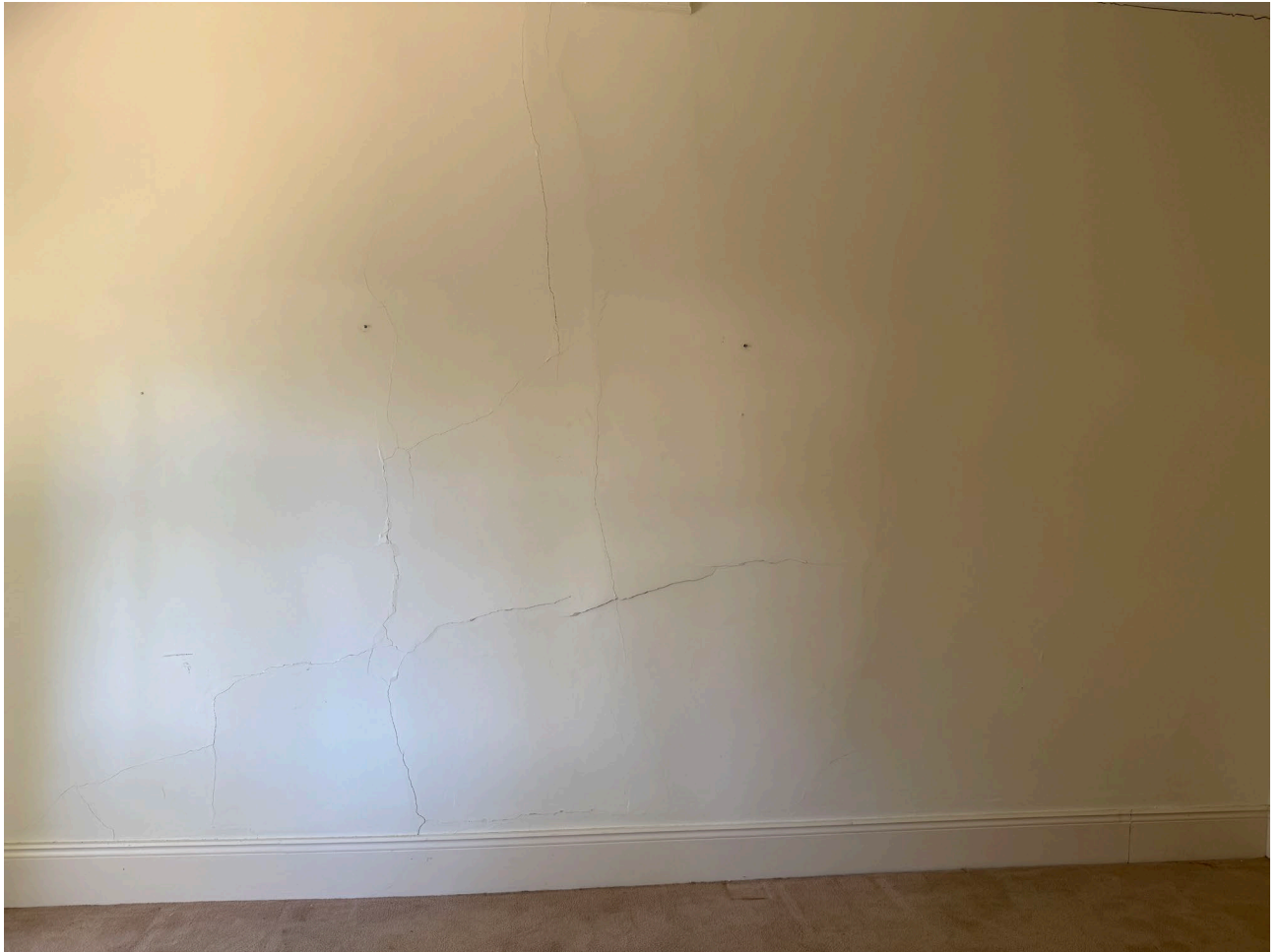
Internal 01 (Damage category 2)
