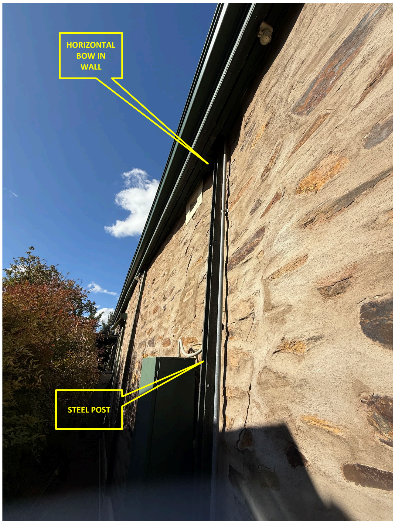
North western wall 06 (Damage category 4)
