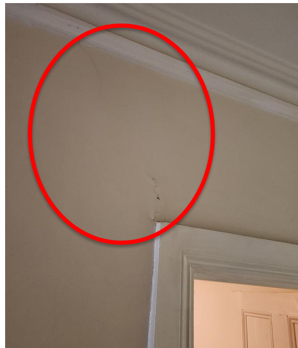
Diagonal cracking above bed 2 door.
