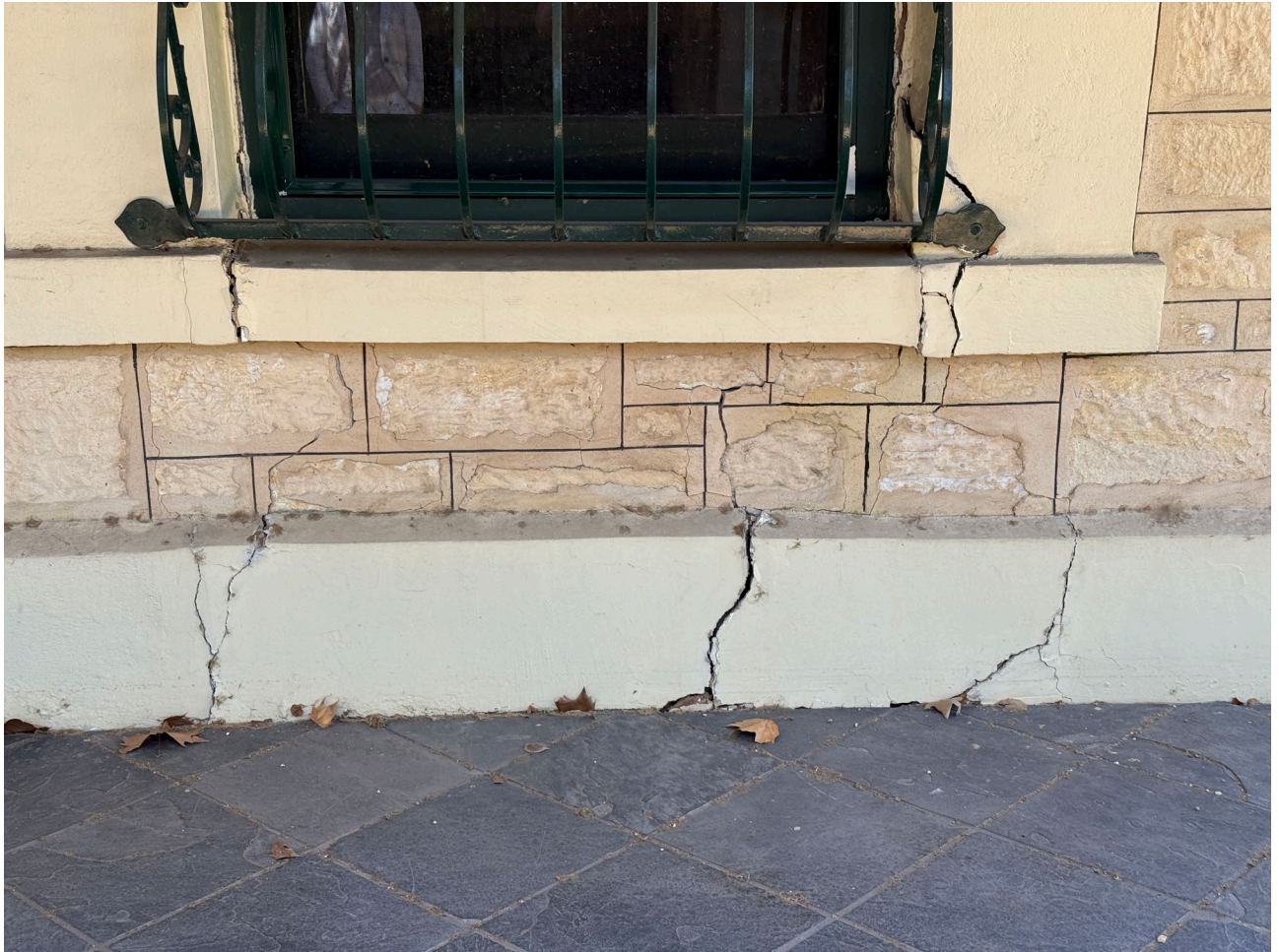
Front wall 02 (Damage category 3)
