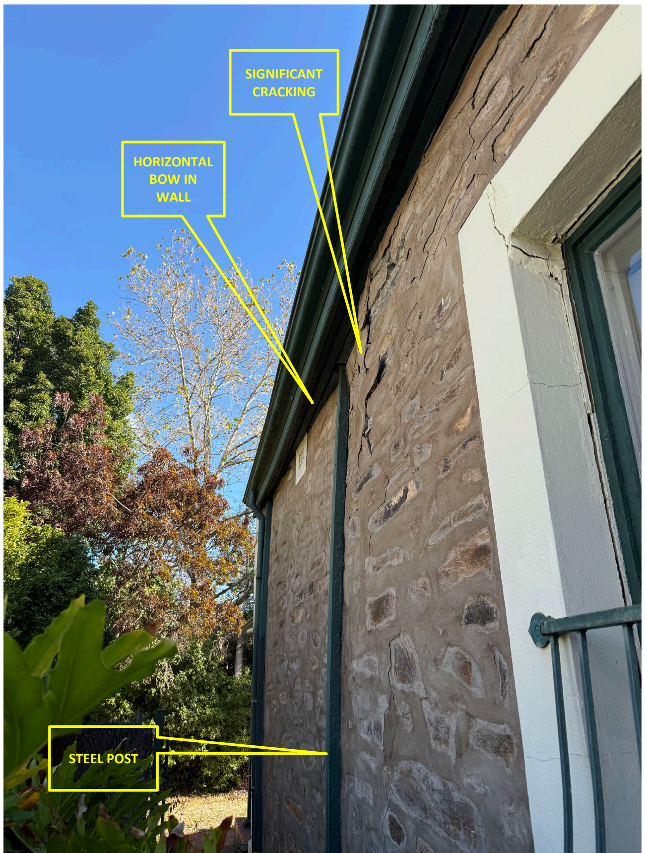
South eastern wall 01 (Damage category 4)
