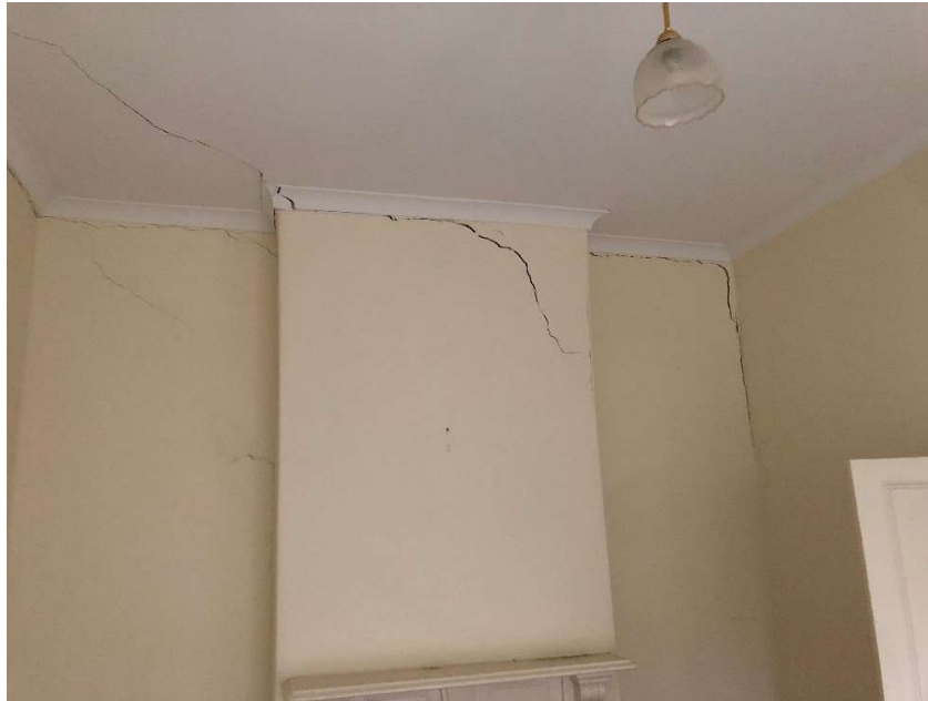
9. Internal view. Major cracking and deformation
