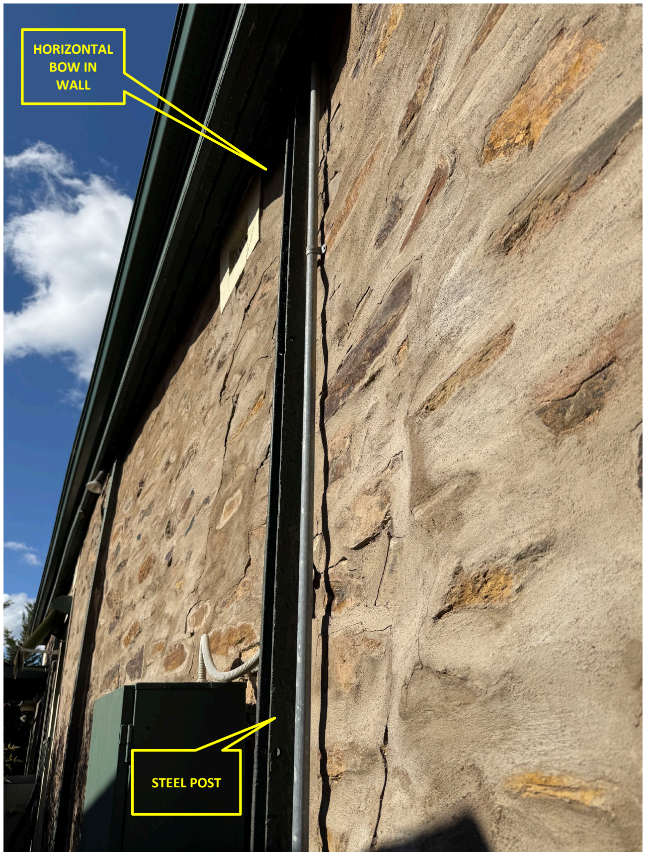
North western wall 07 (Damage category 4)
