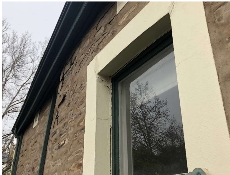
4. South east wall. Severe bowing and cracking deformation of masonry wall
