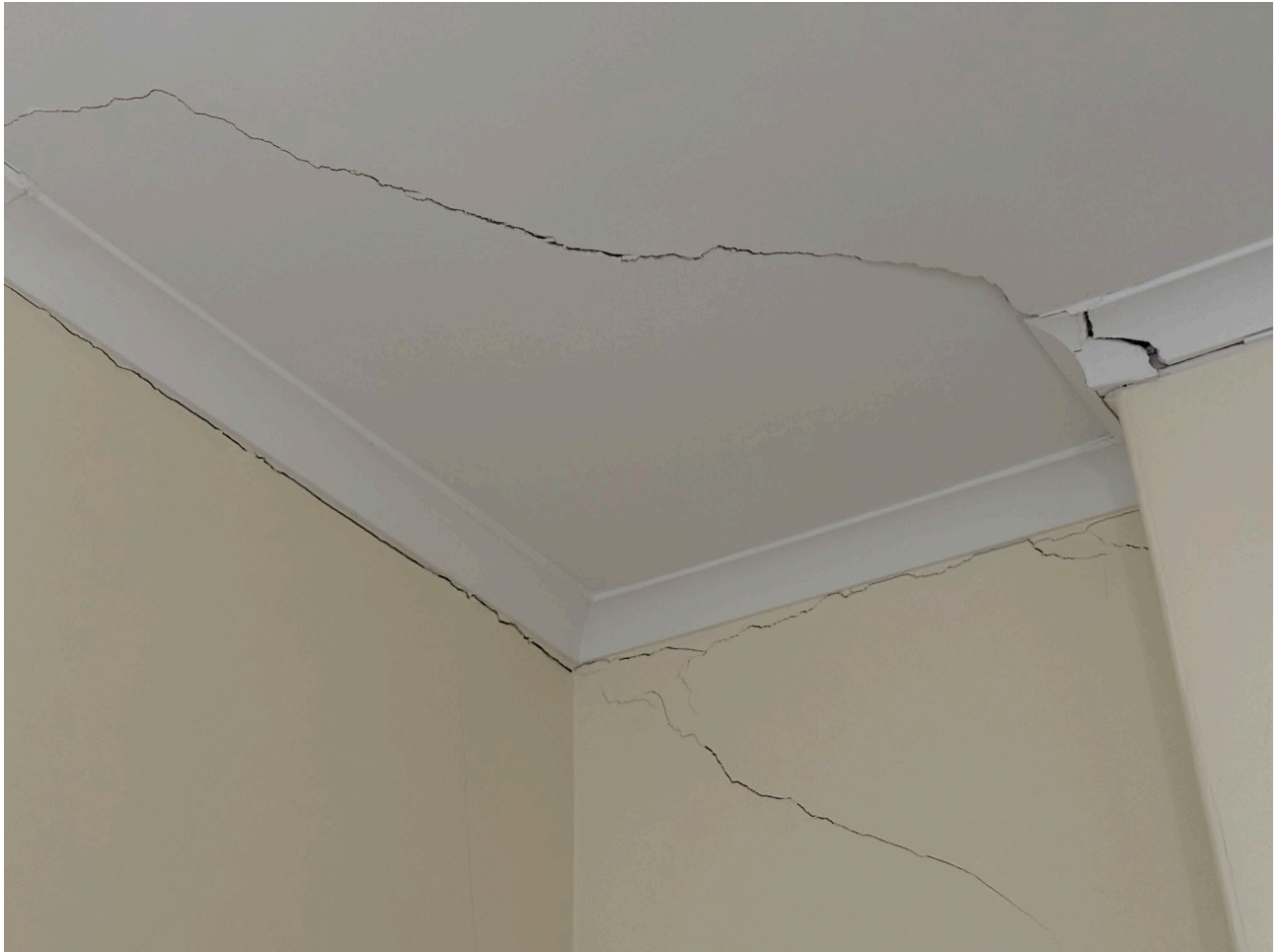
Internal 07 (Damage category 2)
