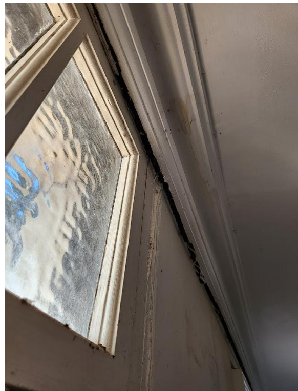
Separation of cornice from southern wall.
