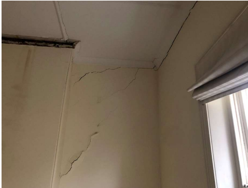
11. Internal view Major cracking and deformation
