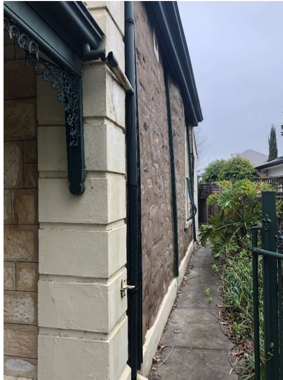
3. South east wall. Steel posts. Severe bowing deformation of masonry wall
