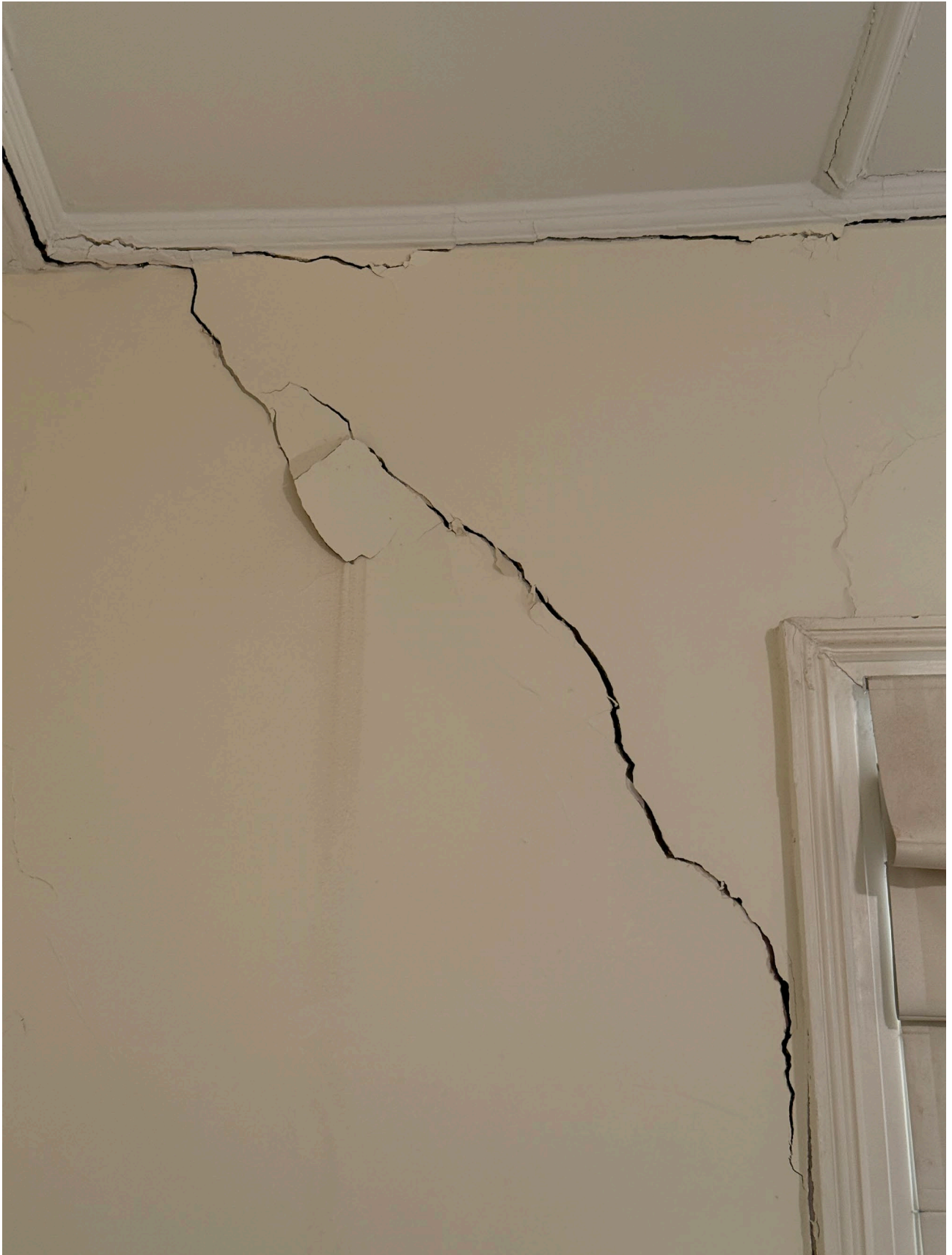
Internal 09 (Damage category 4)
