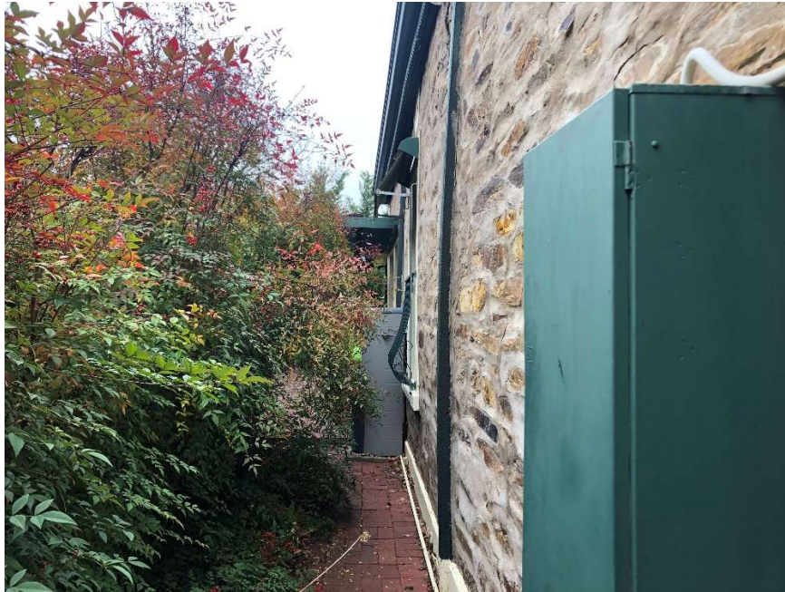
5. North west wall. Steel posts. Horizontal and vertical bowing in masonry
