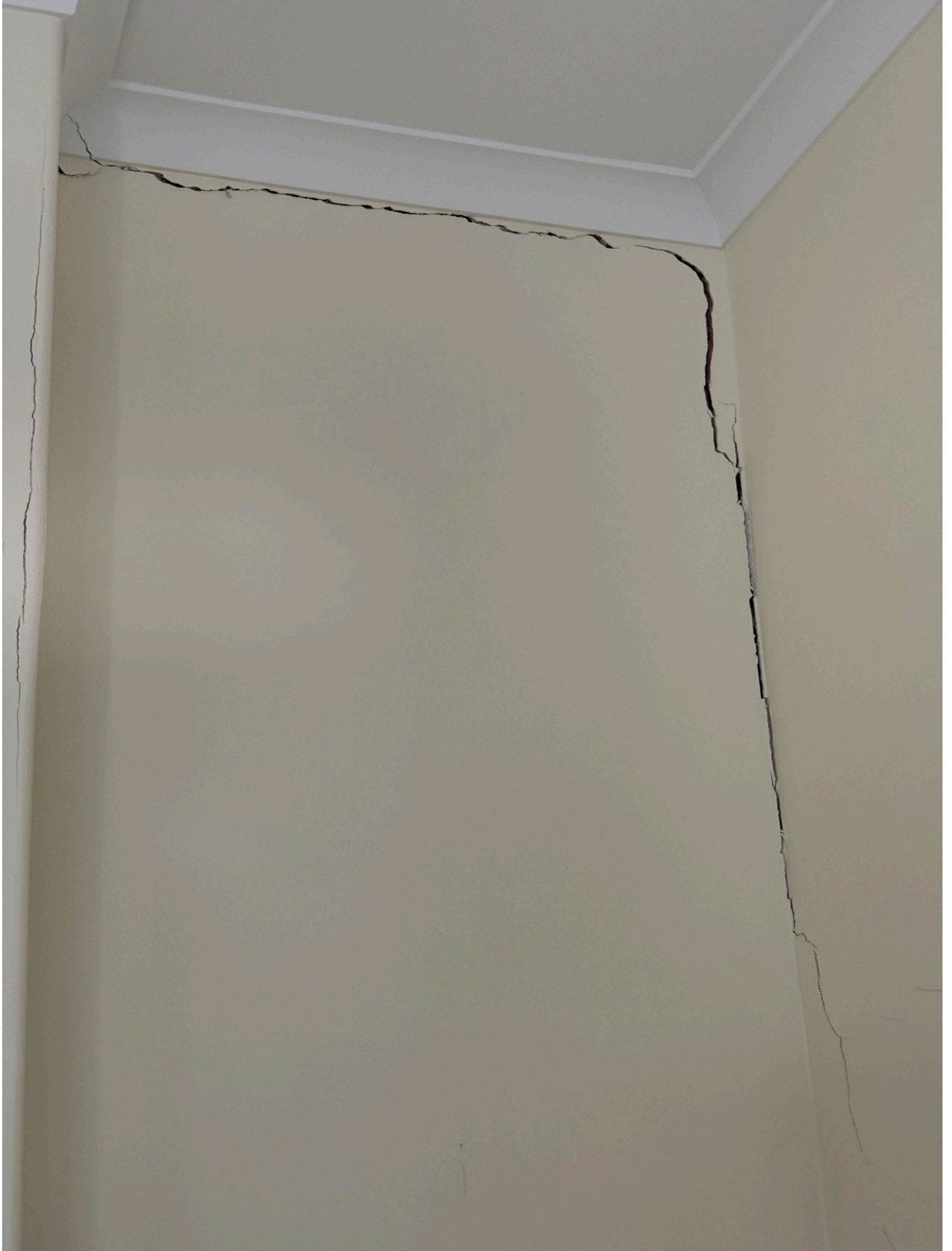
Internal 06 (Damage category 3)
