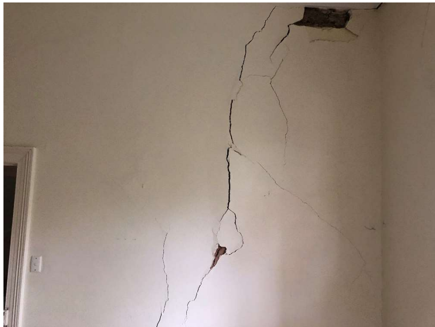
8. Damage category 4 cracking in internal wall.
