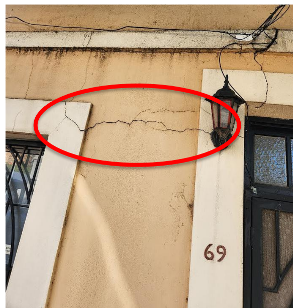
Horizontal cracking west of entry door.
