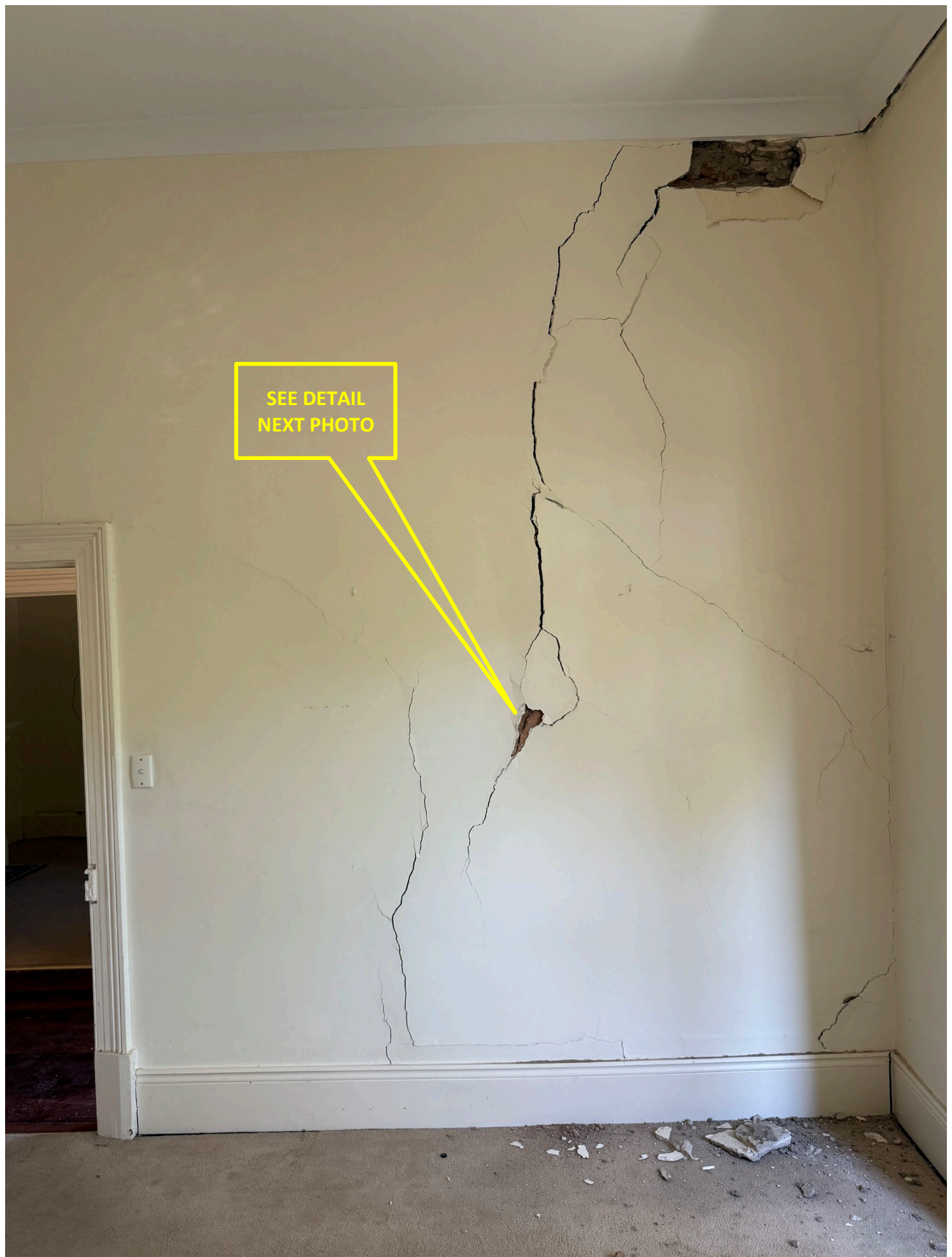
Internal 02 (Damage category 4)
