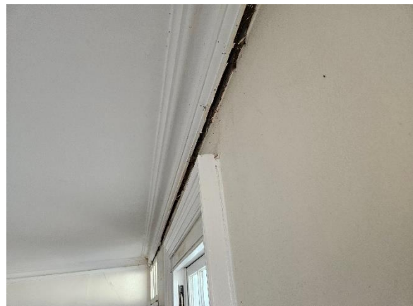
Photo 16 – View of cornice separation along front elevation
