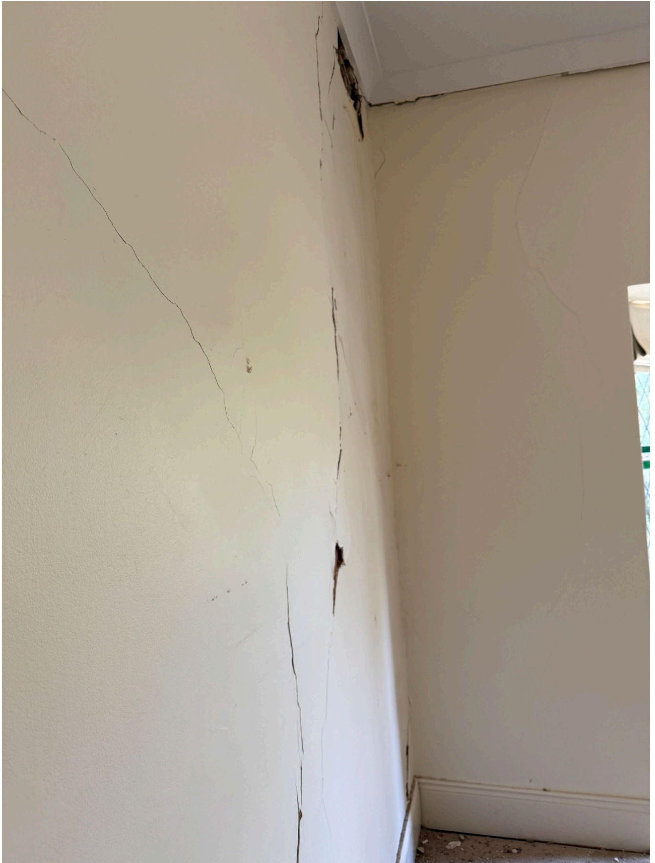
Internal 04 (Damage category 4)
