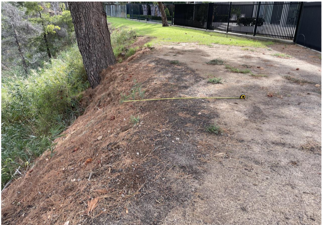
Photo 3.1 Location of possible tension crack (photograph taken 28 May 2025)
