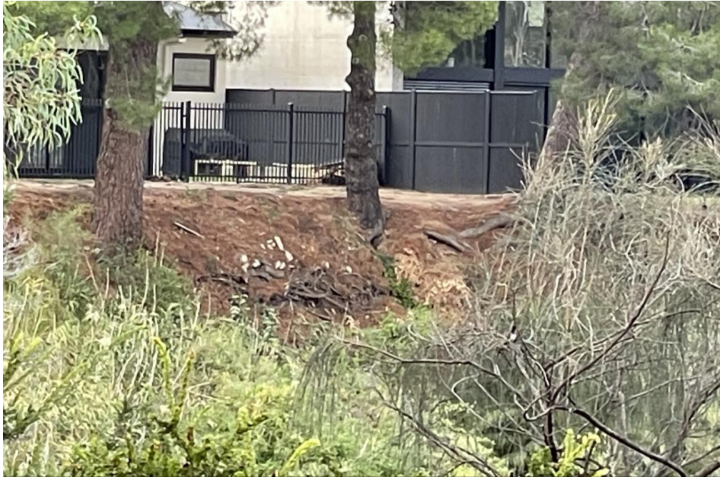
Photo 3.3 Slope at tension crack (photograph taken 28 May 2025)
