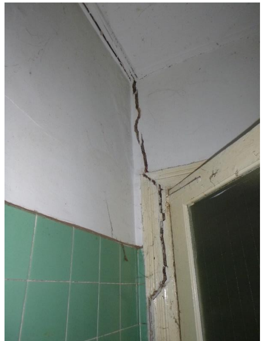
Major cracking – Bathroom
