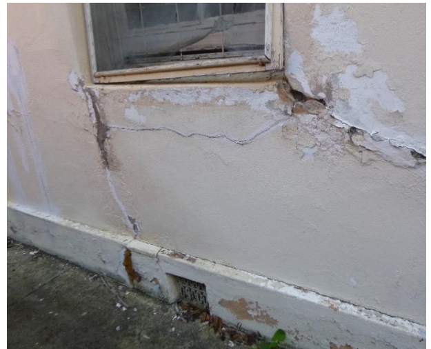
Severe cracking around bedroom 2 window
