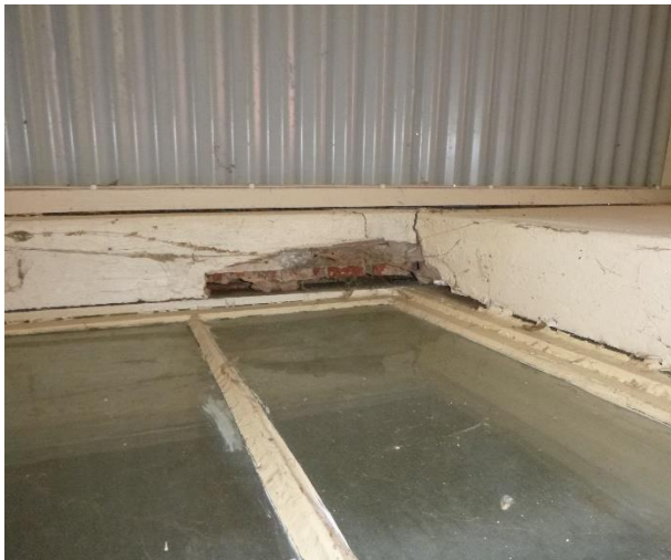
Severe deterioration of brickwork above bedroom 3 window
