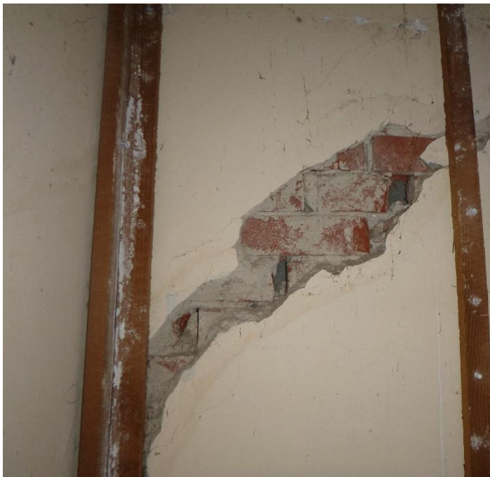
Major cracking – Bedroom 2
