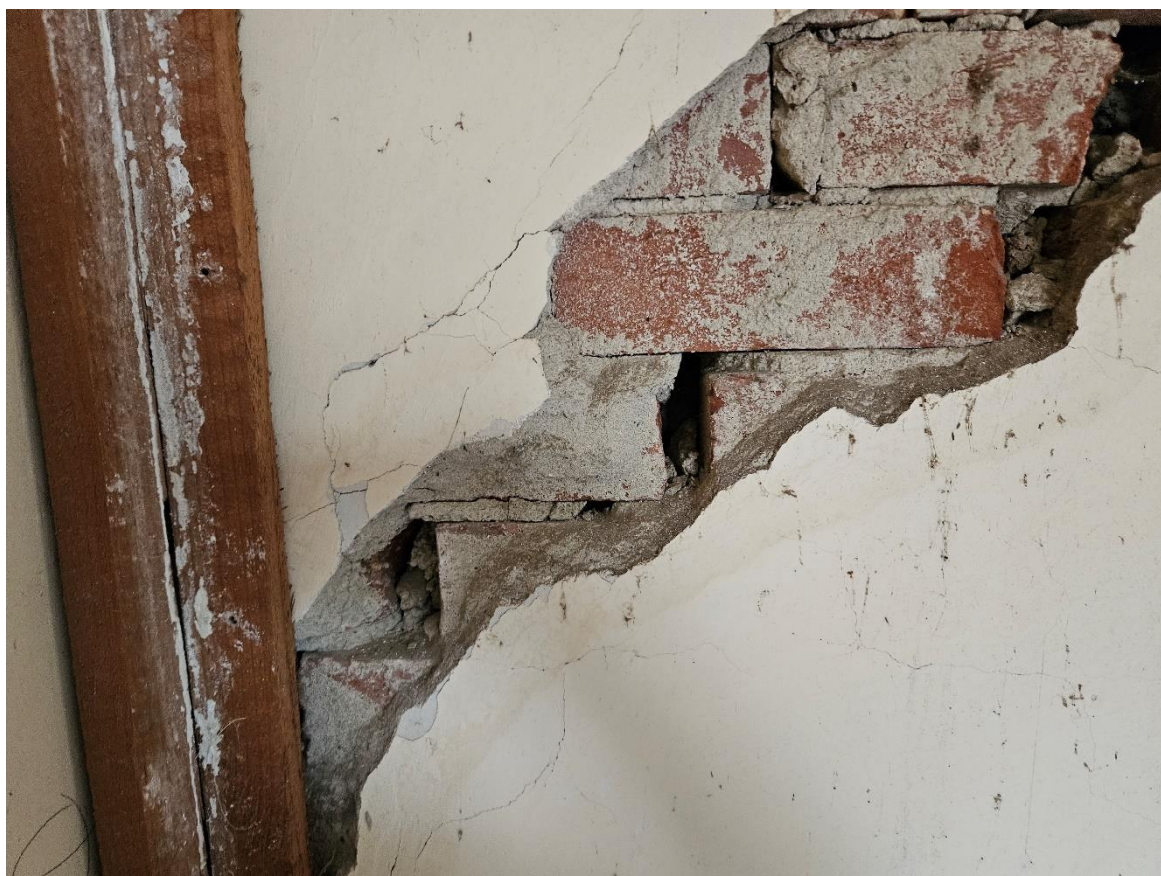
Photo 18 – Cracking to Living room's northern wall
