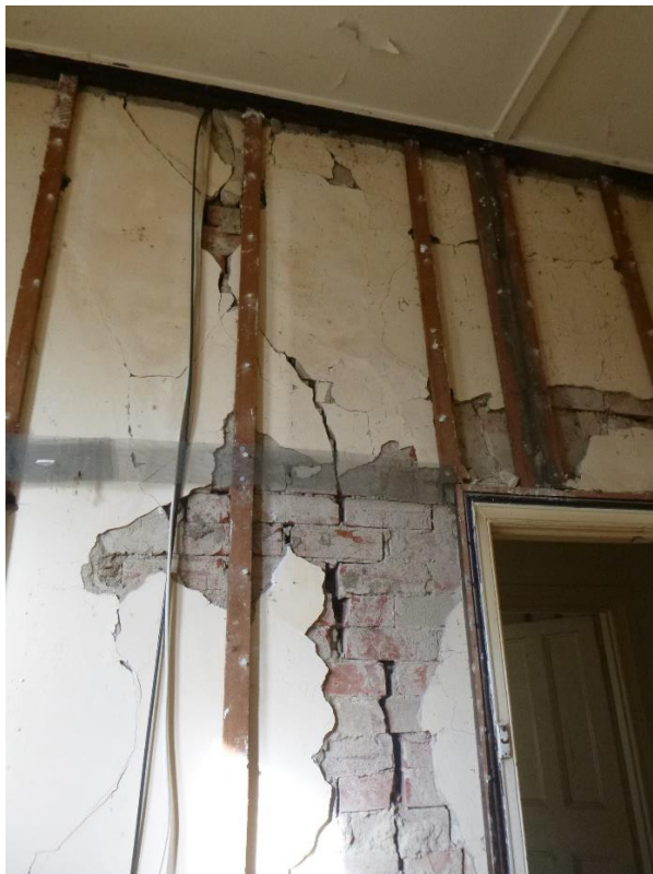
Major cracking – Lounge
