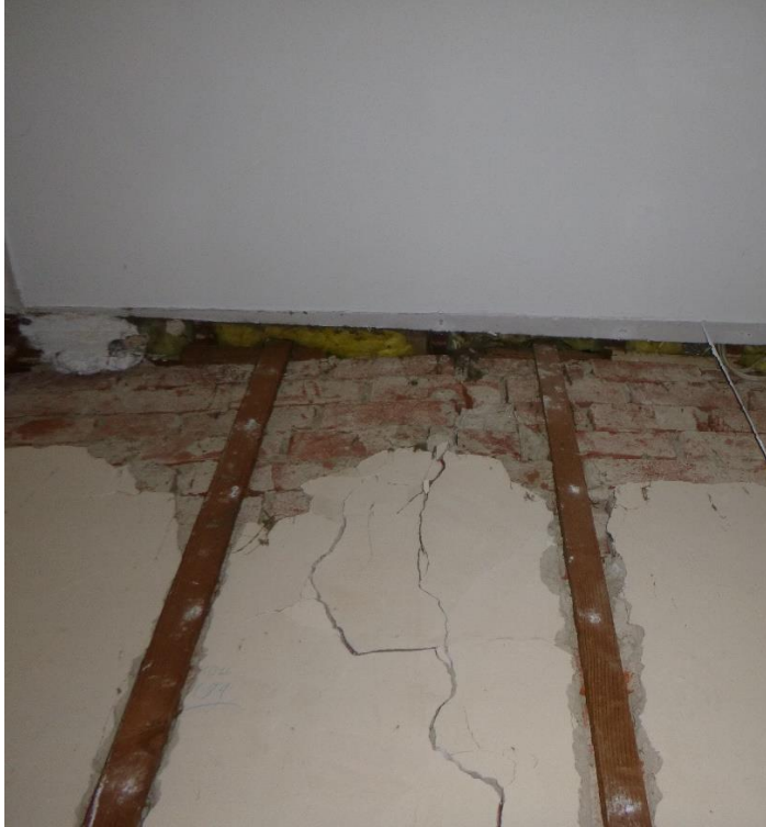
Severe bow in internal wall – Bedroom 1
