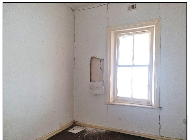
Photo 5 – Typical cracking to internal plasterboard claddings
