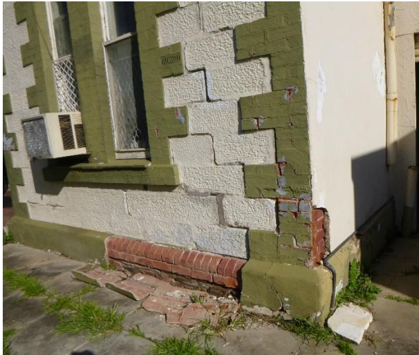
Major cracking and deterioration in north-eastern corner
