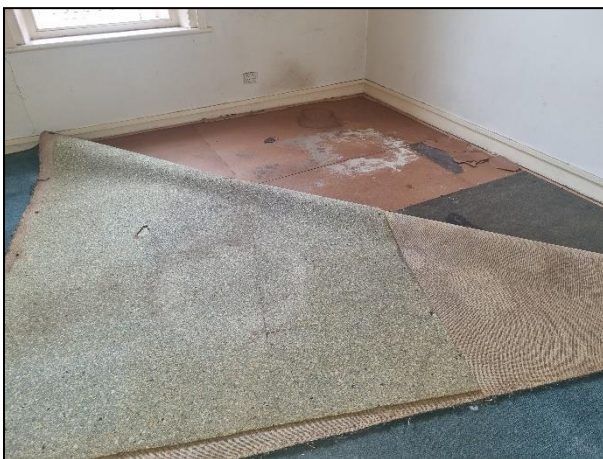
Photo 4 – Dropped floor in south-western room
