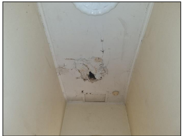
Photo 11 – Collapsed plaster ceiling due to roof leak
