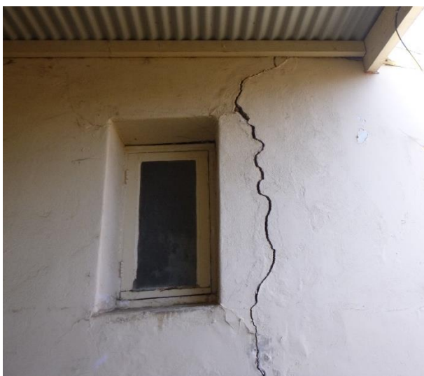
Major cracking between main house and lean-to
