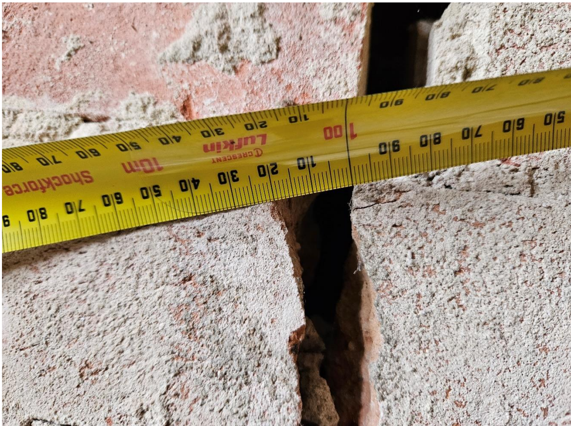
Photo 2 – Close up of crackingshown in Photo 1
