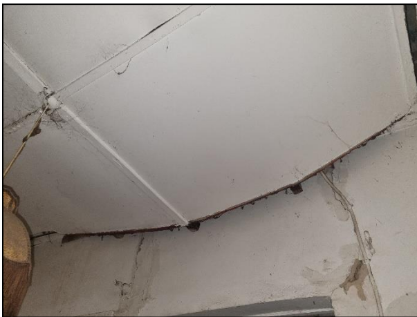
Photo 10 – Collapsed ceiling to rear addition
