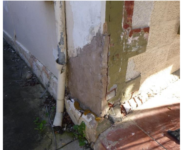
Severe deterioration in south-eastern corner
