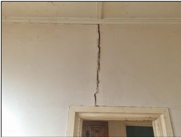
Photo 2 – Severe structural cracking to internal wall
